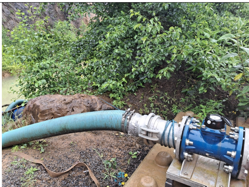
Fig 2: Meter with pump visible in the background
