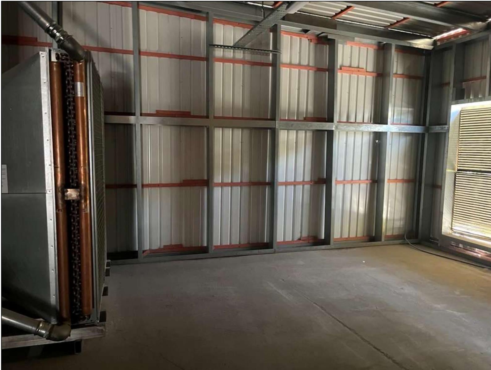
Figure 6: Attenuator required to the inlet of the Biomass to achieve a maximum permissible sound pressure level of 85dB L_{Aeq,T}
