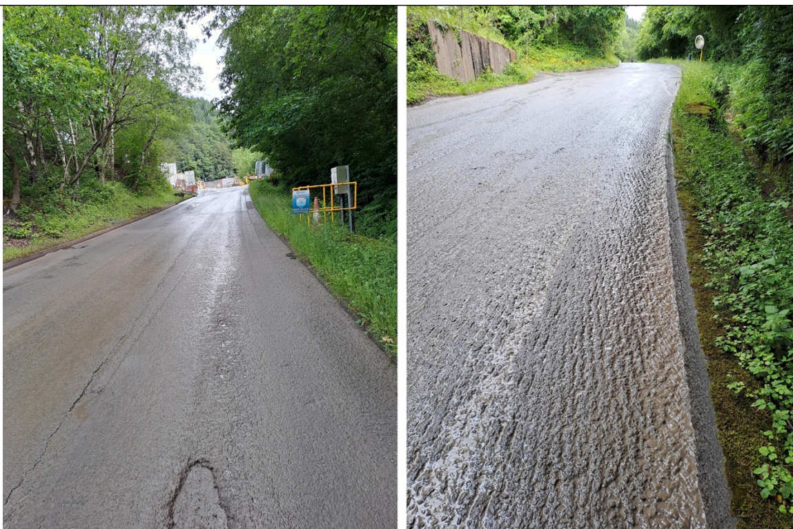
Figure 11 – The conditions of the road as observed during the visit.
