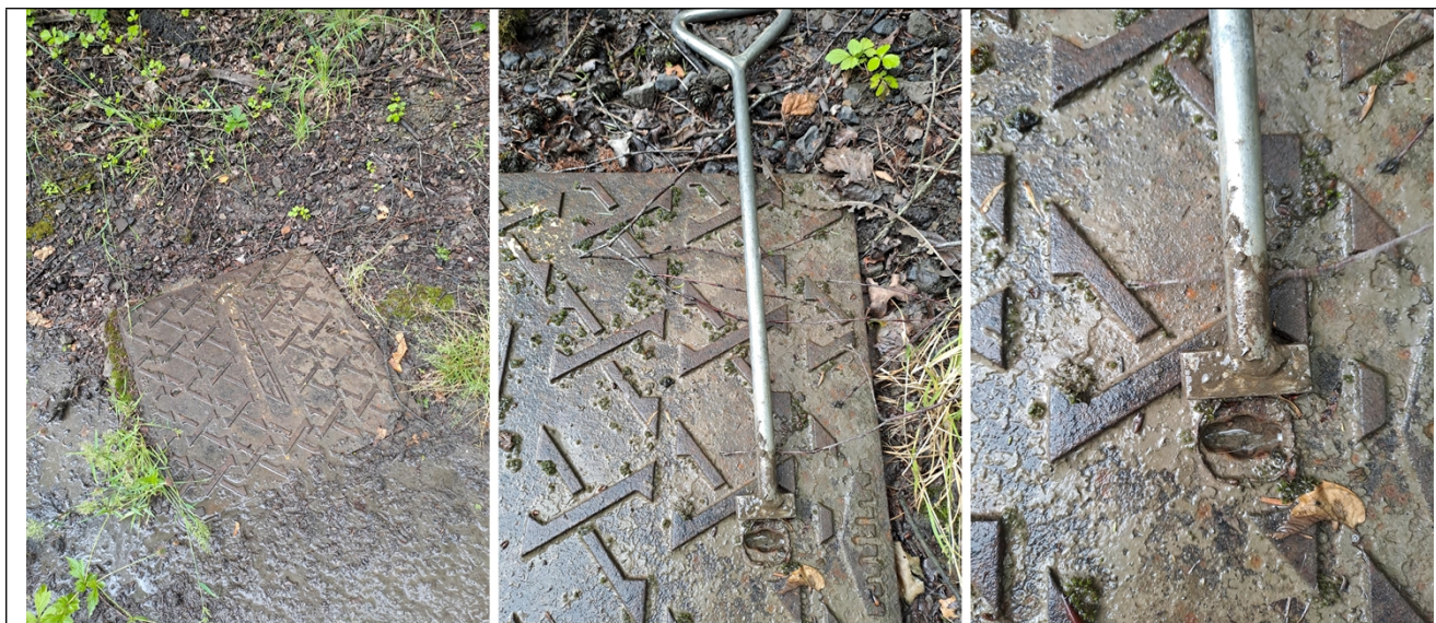
Figure 15 – The chamber identified as Silt Trap 3 which we were unable to be lifted during the visit.
