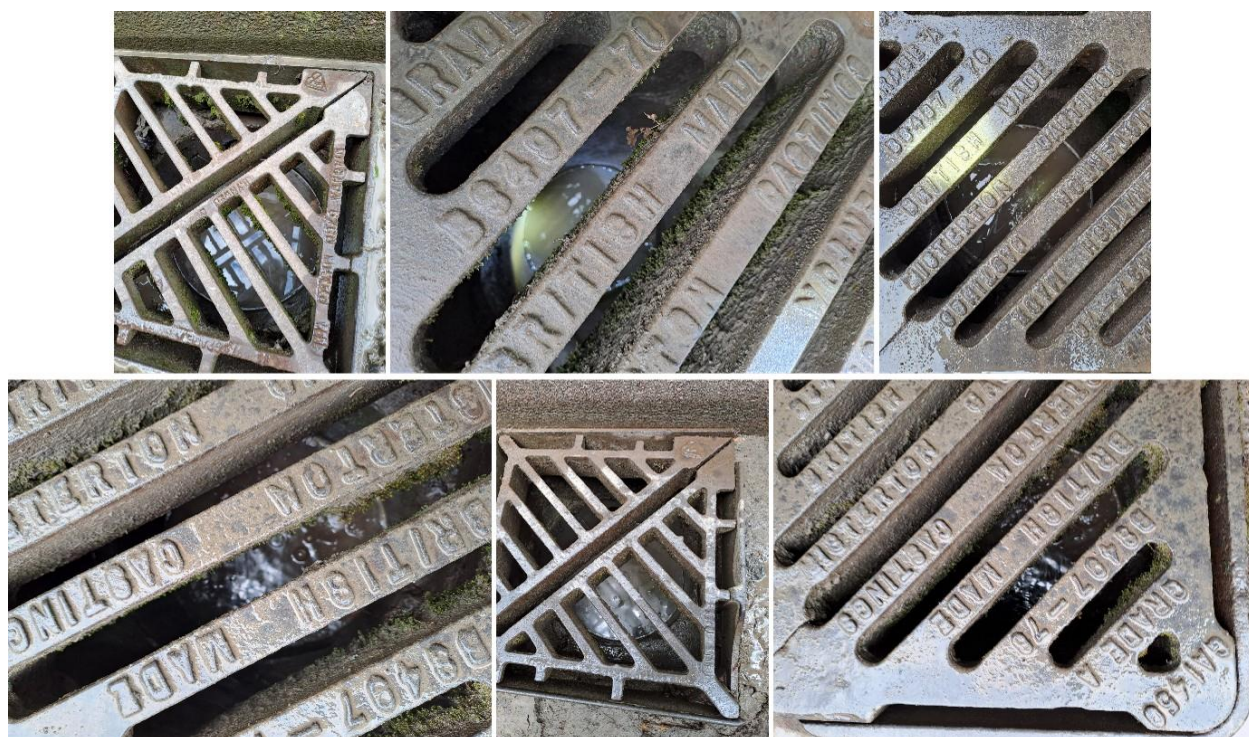
Figure 13 – The condition of the road gullies as observed during the visit.
