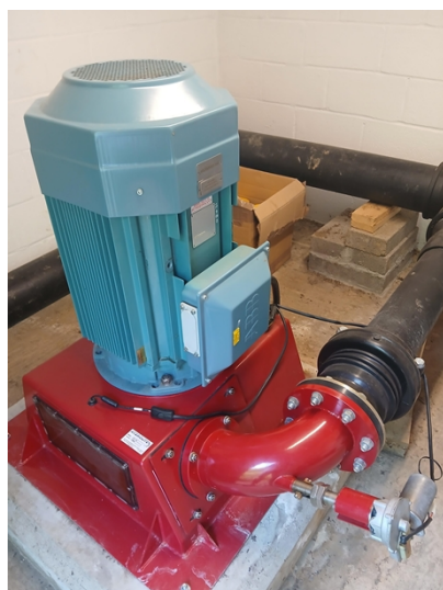
Fig 5 - Pump house turbine
