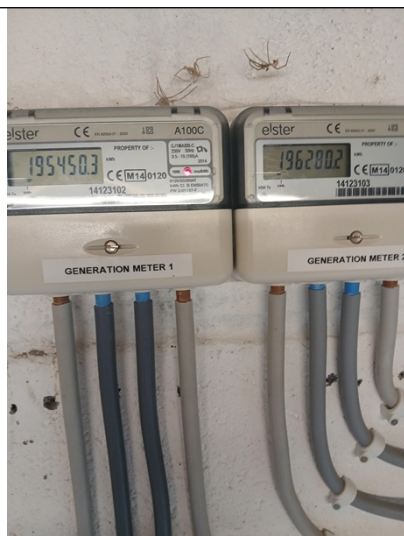
Fig 4 - Pump House meters
