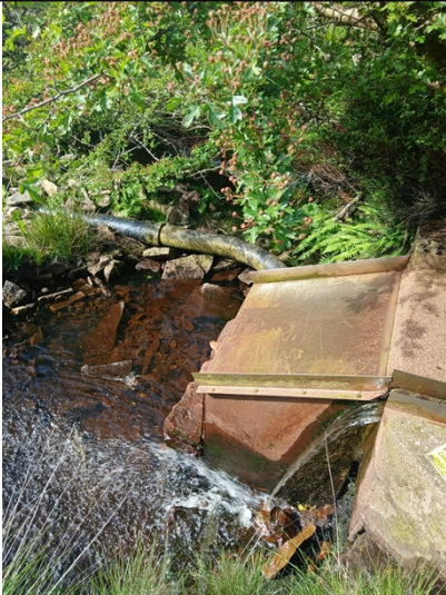
Fig 2 - Concrete Weir, Screen, Hands Off Flow Notch and gravity fed Pen Stock
