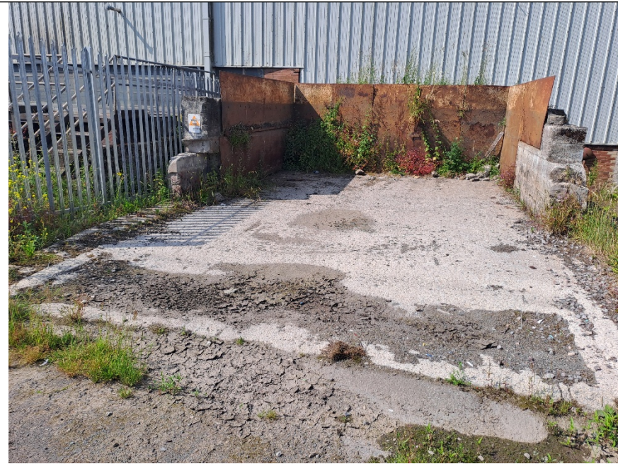
Image 1 shows the dewatering bay for the site's permitted activity. The bay has not been operational since mid-2025.
