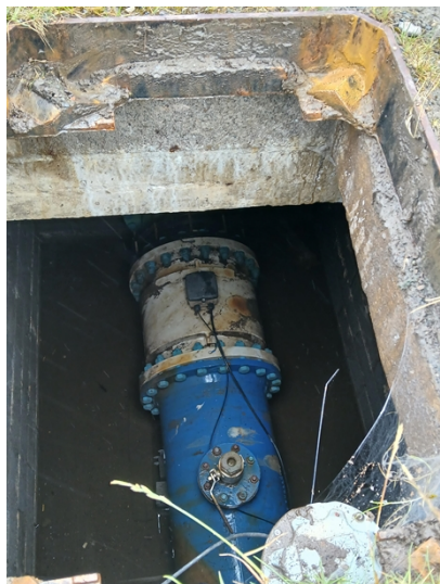
Fig 5 - Metering in place
