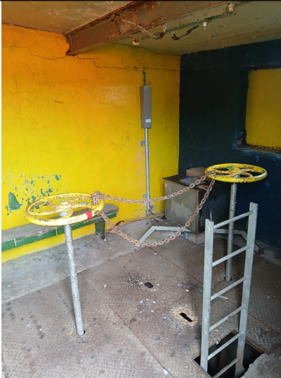
Fig 3 - Scour valve and telemetry
