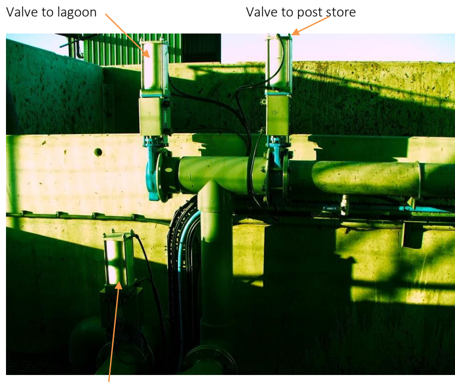
Valve to Grit Trap Sump
