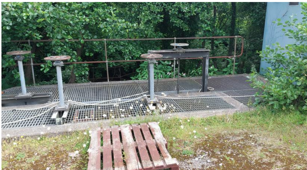
Photograph 9-3: Effluent outfall diversion chamber
