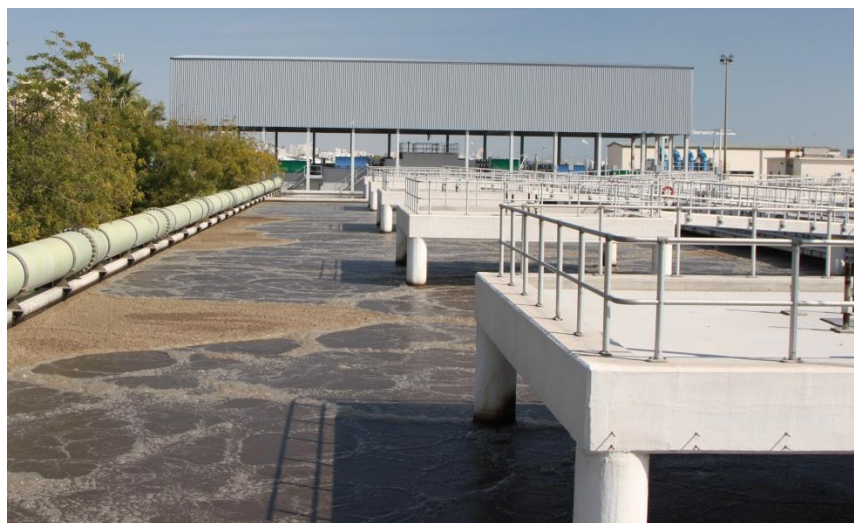
Figure 7: One of the two aeration lanes converted to HYBACS, with SMART unit building in the background
