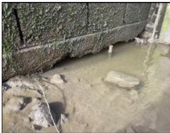
Figure 4: Scour Damage to culvert wingwall.
