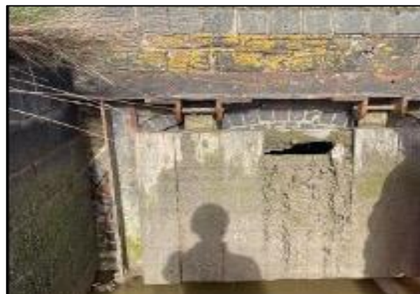
Figure 7: Damaged tidal flap.
