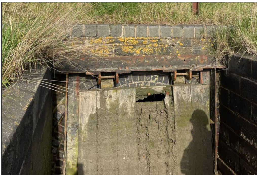
Figure 2: Damaged Tidal Flap.
