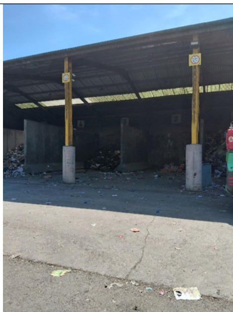
Image 3: Concrete block segregation bays inside the waste transfer station building.
