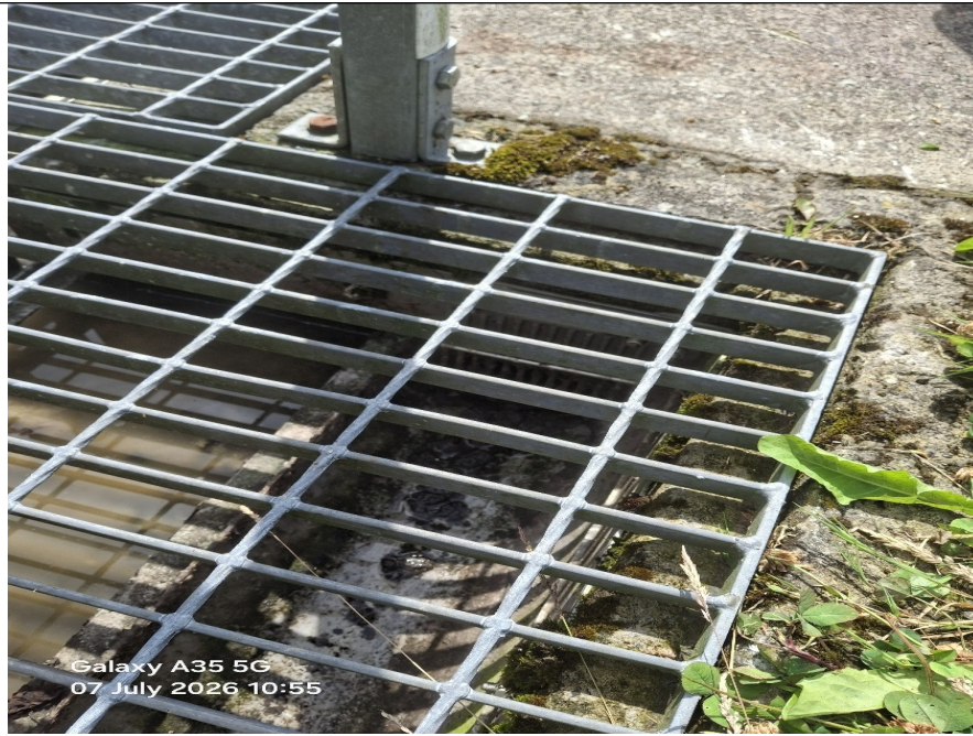
Figure 2 Bar screen on the storm overflow
