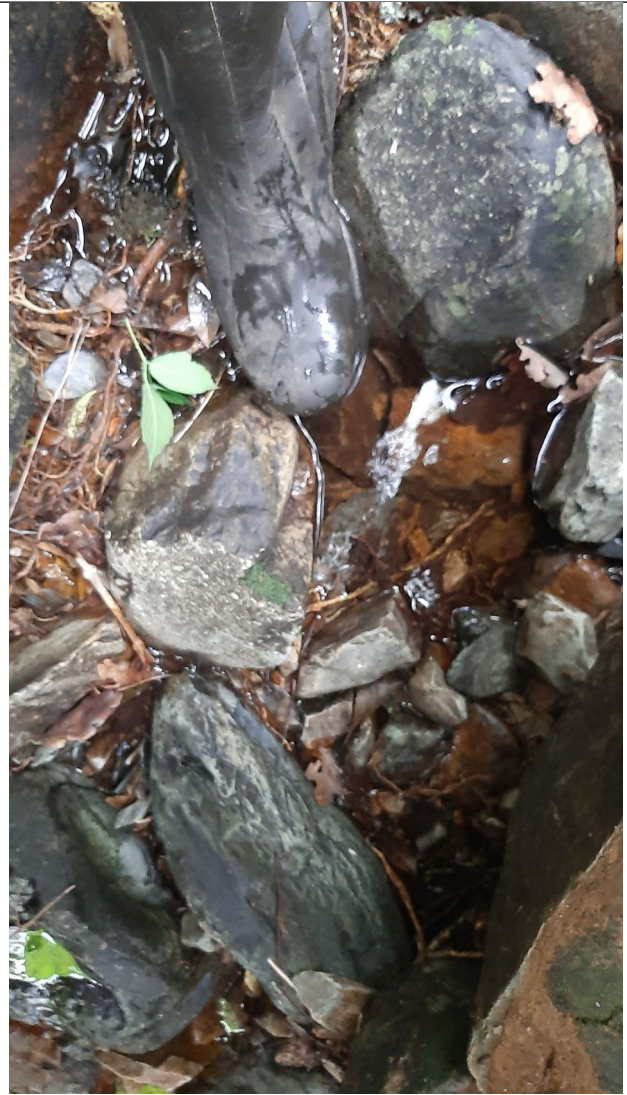
Figure 18 -Bed substrate beneath bridge
