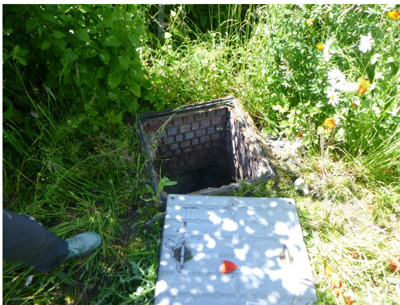
Photograph 3: Effluent sample point at SJ 21842 00246
