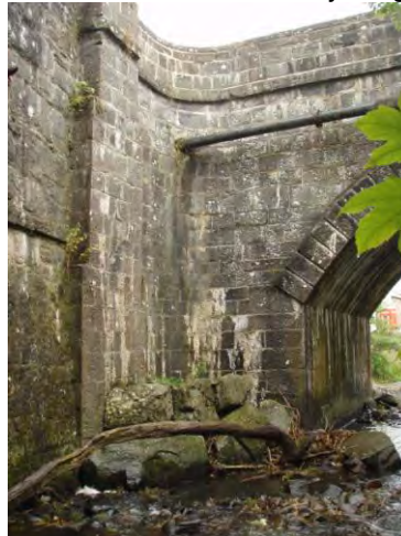
Plate 4 Site 2– Boulders by bridge
