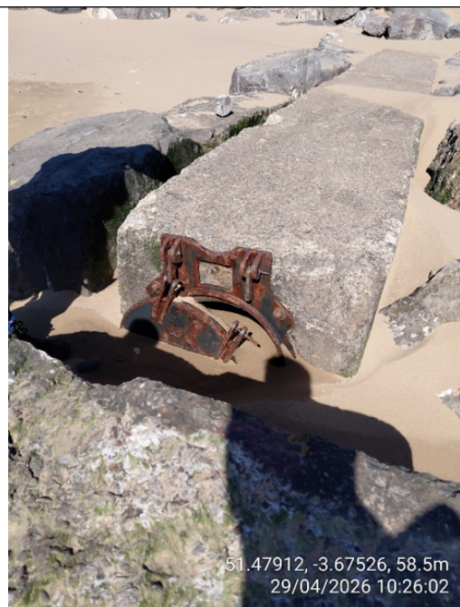
Photograph 2: Point of Discharge
