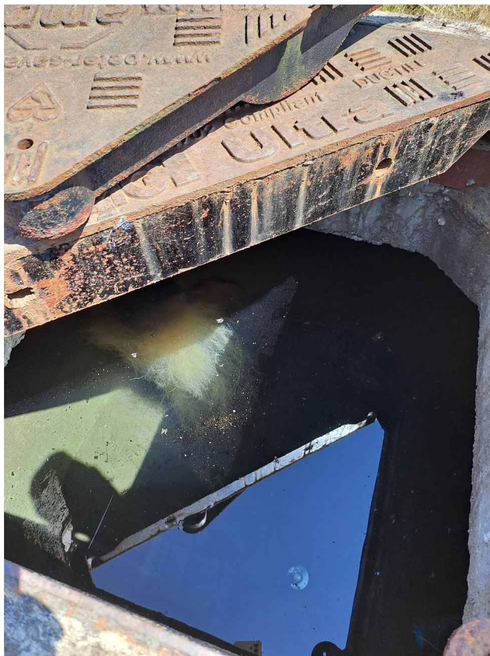
Figure 2 – The catch tank (with root ingress visible) as observed during the inspection.
