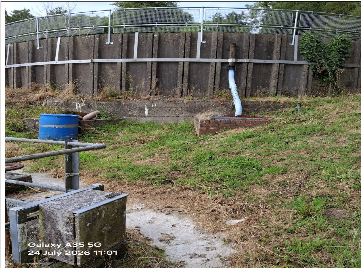
Figure 1, Metal brace fitted around the filter bed.
