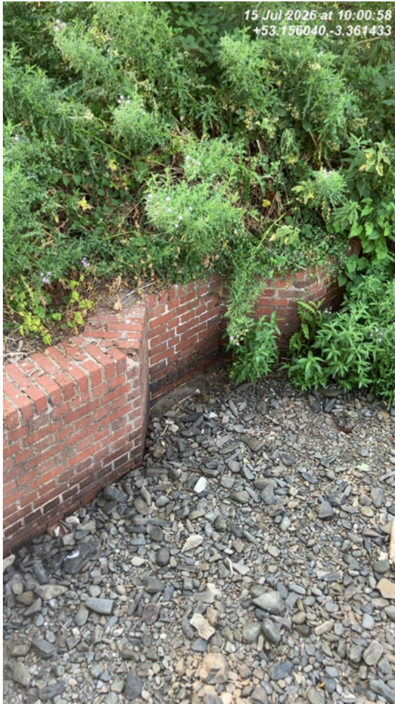
Figure 2. Photograph of the blocked outfall, taken at 10:00 on 15 July 2026.
