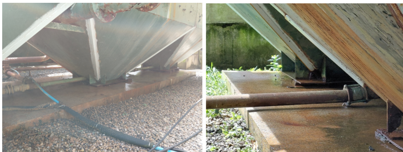
Image 4 & 5: Losses noted beneath the Clarifiers.
