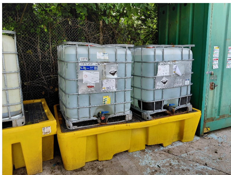
Image 7: Ferric Chloride and Sodium Hydroxide (Caustic Soda) storage bunds
