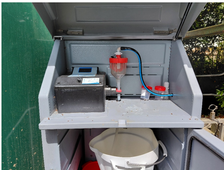
Image 6: View of internal components of Hach Lange Bühler Autosampler
