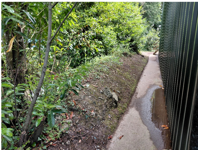
Image 3: Proximity of earth banking bordering the Afon Bran to the concrete blockwork wall associated with the DAF Plant.
