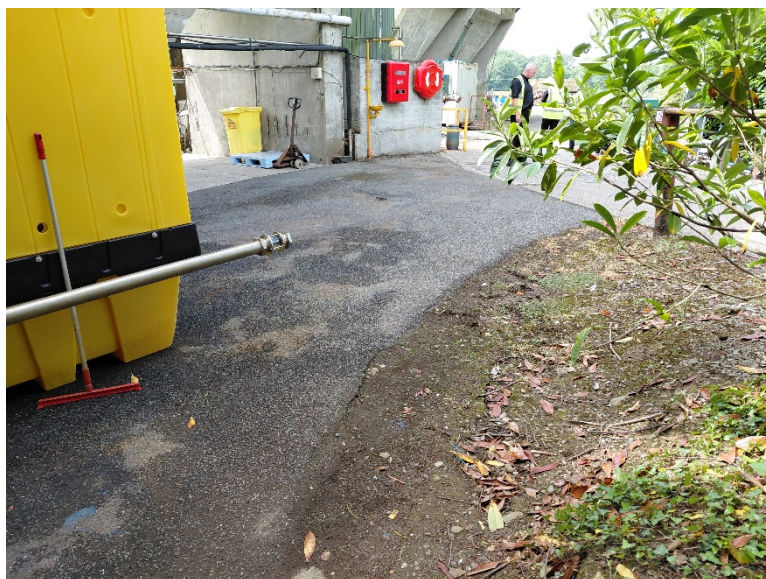
Image 2: DAF pipework extending beyond curtilage of partially bunded area
