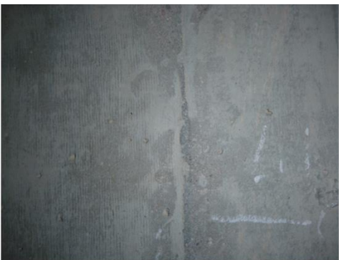
Figure 4: Site imperfections (<0.5m)
