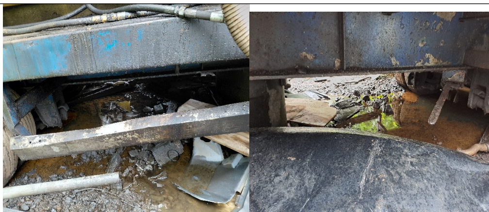
Photo 7 & 8 showing drip tray underneath the crusher/baler
