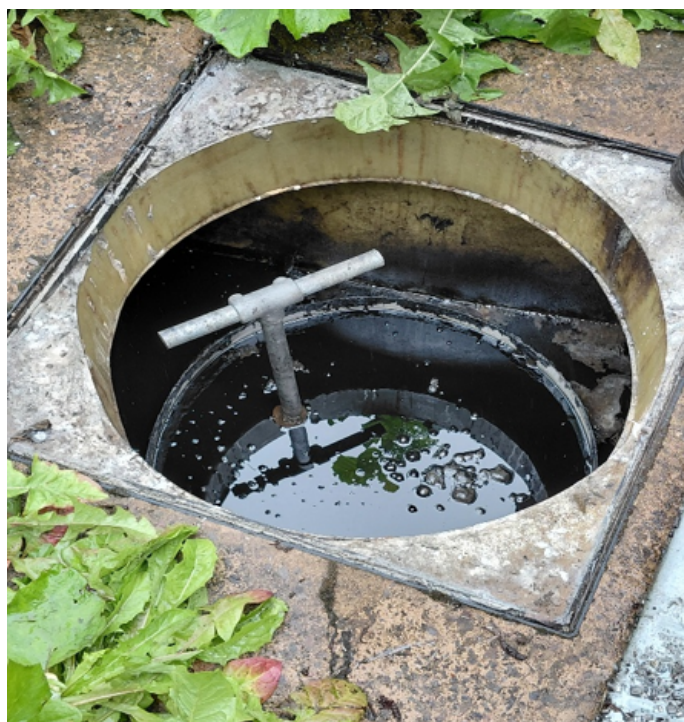
Photo 1 - inspection chamber of the interceptor high level of liquid
