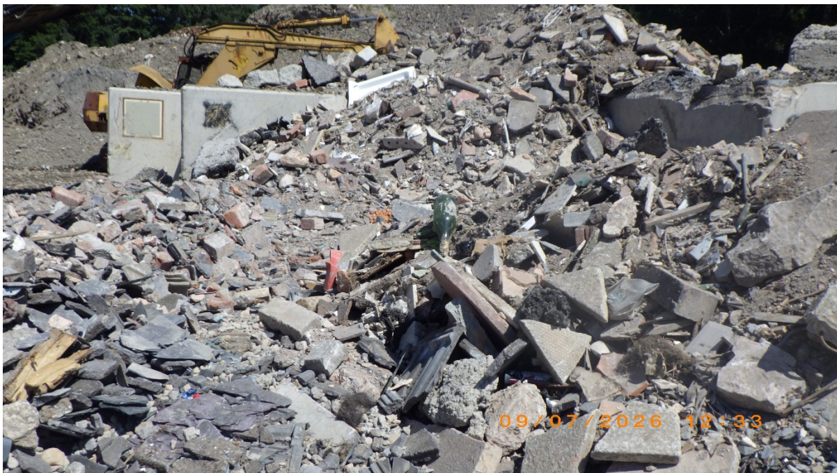
Plastic and glass contaminants seen on site
