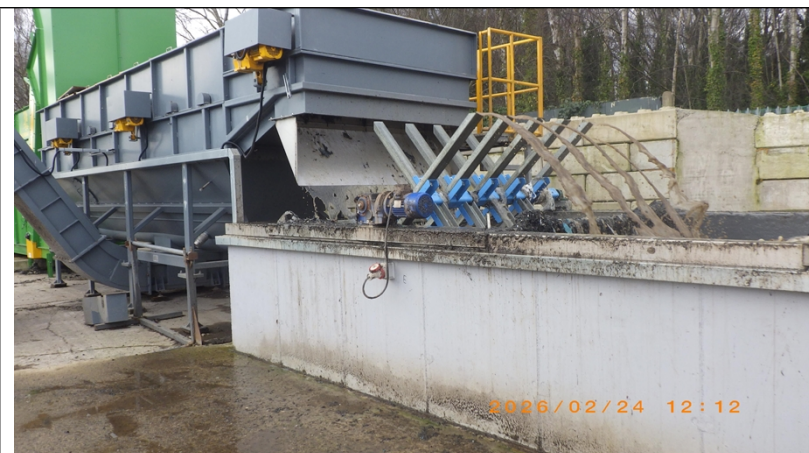
Photograph of one of three new wash baths installed in total. These are not listed on the current site plan incorporated into the permit.
