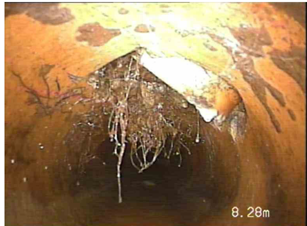
2, 00:02:00, 8.28 m Connection defective, connecting pipe is intruding at 1 o'clock, 100mm dia, intrusion: 10%
