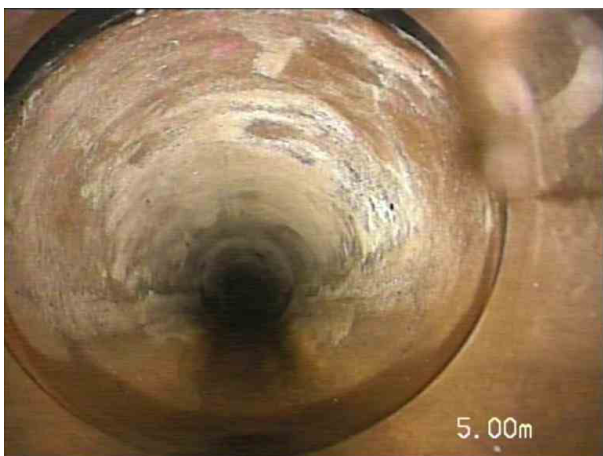
3, 00:00:55, 5.00 m Joint displaced, large
