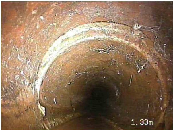
1, 00:00:29, 1.33 m Joint displaced, large
