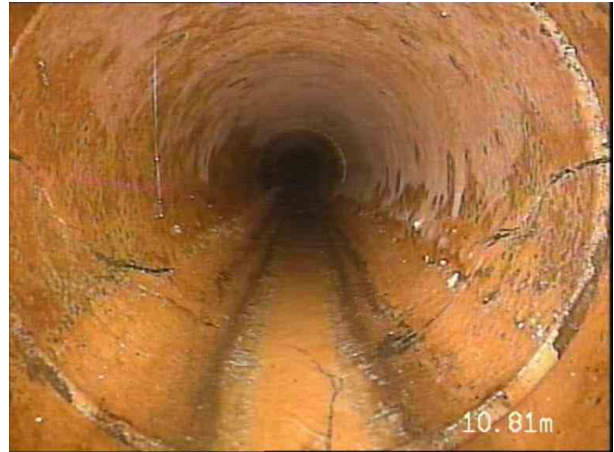
2, 00:01:19, 10.81 m Fracture, longitudinal at joint at 6 o'clock
