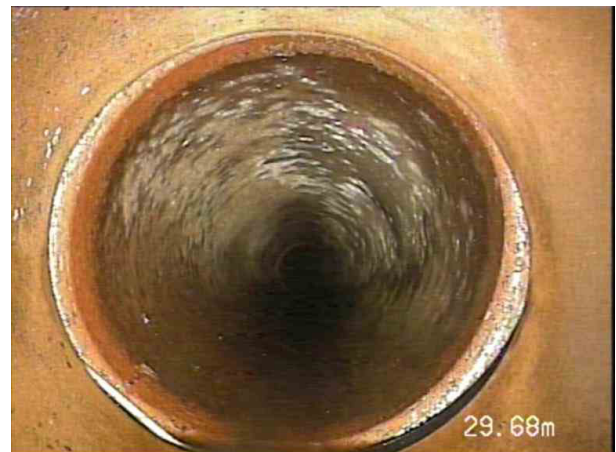
18, 00:05:26, 29.68 m Open joint, large
