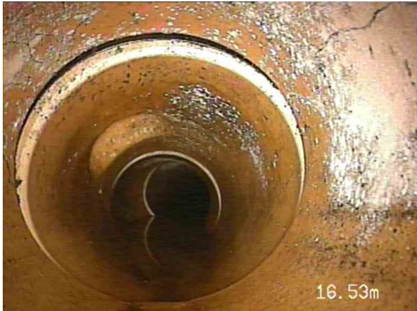
1, 00:02:37, 16.53 m Joint displaced, large
