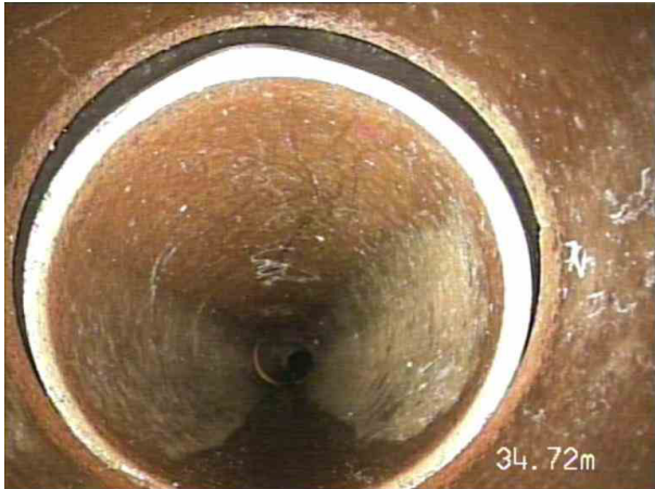
19, 00:05:57, 34.72 m Open joint, large
