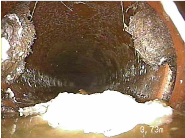
1, 00:00:47, 3.71 m Roots, mass at joint, 20% cross-sectional area loss
