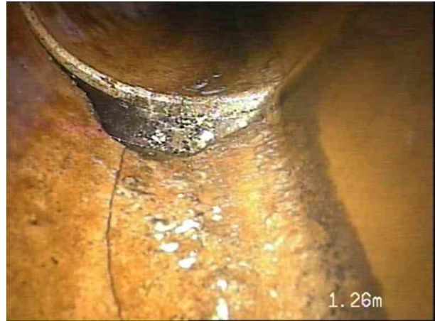
2, 00:00:31, 1.26 m Hole in drain or sewer from 7 o'clock to 8 o'clock
