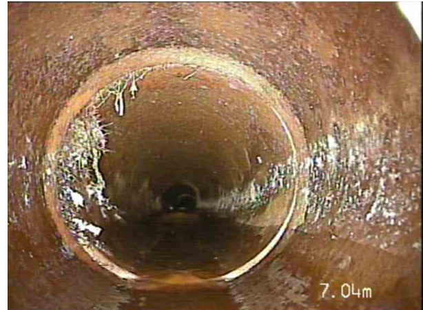
2, 00:01:16, 7.00 m Roots, mass at joint, 10% cross-sectional area loss
