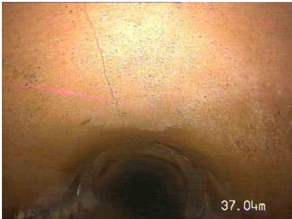
7, 00:05:28, 37.04 m Crack, longitudinal at 12 o'clock
