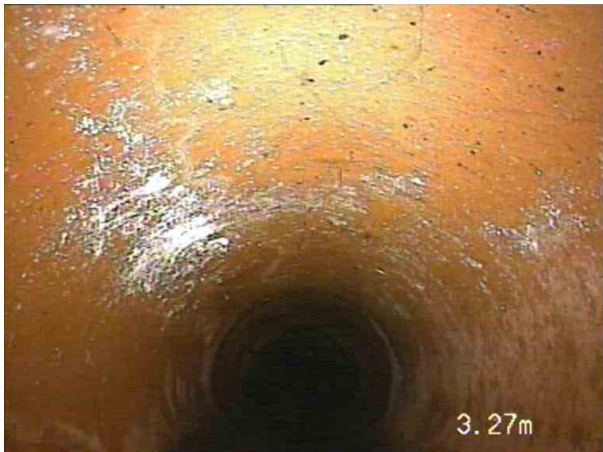
1, 00:00:36, 3.27 m Crack, longitudinal at 12 o'clock
