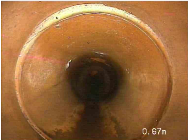
1, 00:00:17, 0.67 m Crack, circumferential at joint from 10 o'clock to 3 o'clock
