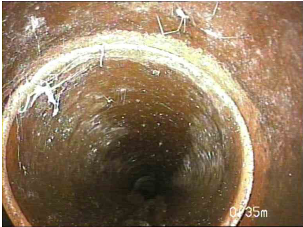
1, 00:00:19, 0.35 m Open joint, large
