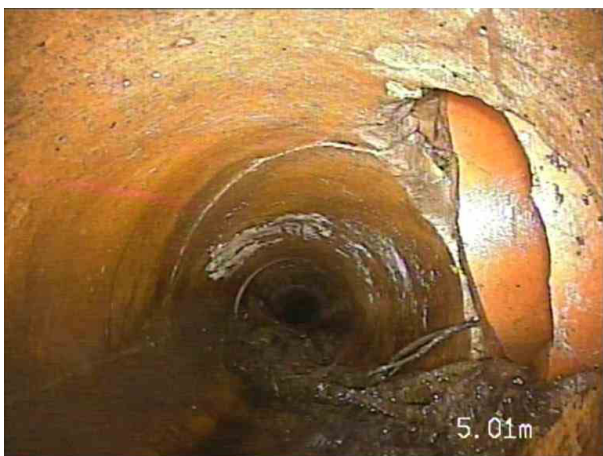
3, 00:01:12, 5.01 m Connection defective, connecting pipe is intruding at 2 o'clock, 150mm dia, intrusion: 10%
