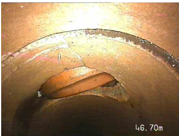
9, 00:06:33, 46.70 m Crack, longitudinal at joint at 12 o'clock
