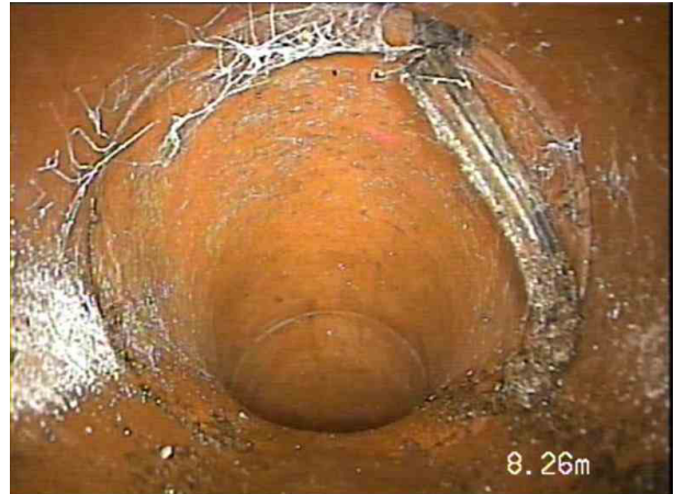
2, 00:01:19, 8.26 m Sealing ring intruding from 12 o'clock to 4 o'clock
