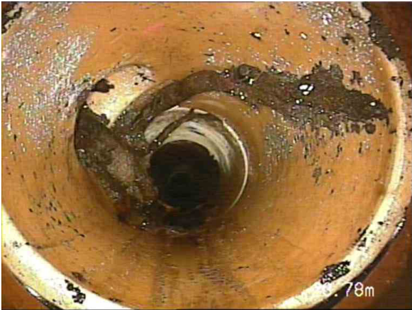
13, 00:04:23, 23.78 m Joint displaced, medium
