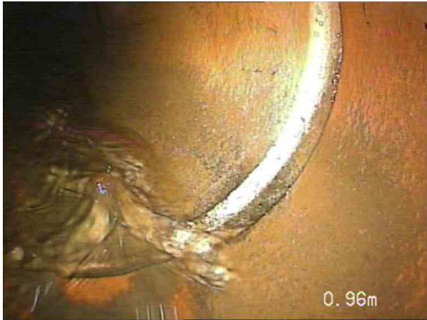
1, 00:00:21, 0.96 m Open joint, large
