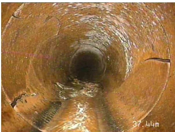
3, 00:03:57, 37.44 m Fracture, spiral at joint from 3 o'clock to 7 o'clock
