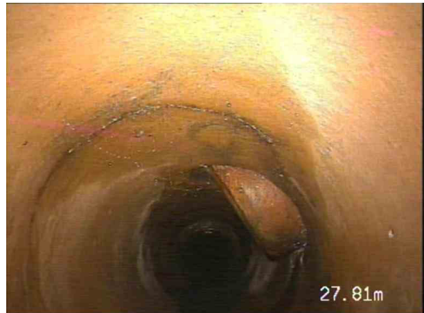
4, 00:03:49, 27.81 m Fracture, spiral from 8 o'clock to 2 o'clock
