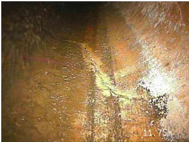
3, 00:02:32, 11.75 m Cracks, spiral from 3 o'clock to 6 o'clock
