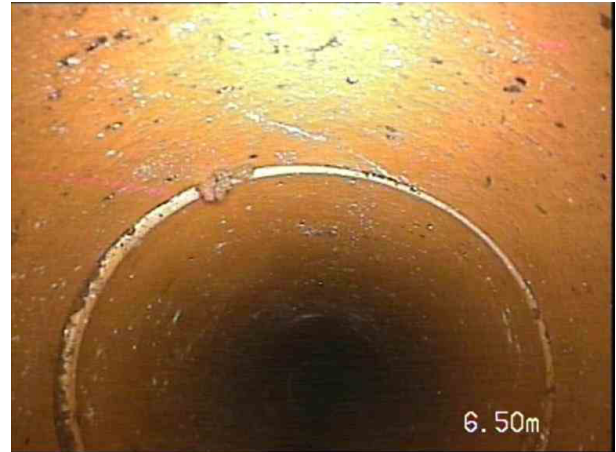
2, 00:01:07, 6.50 m Crack, longitudinal at joint at 12 o'clock
