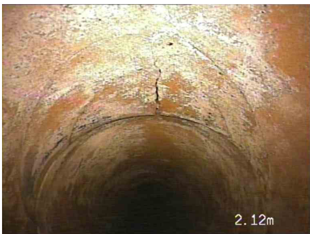
3, 00:00:57, 2.12 m Fracture, longitudinal at joint at 12 o'clock
