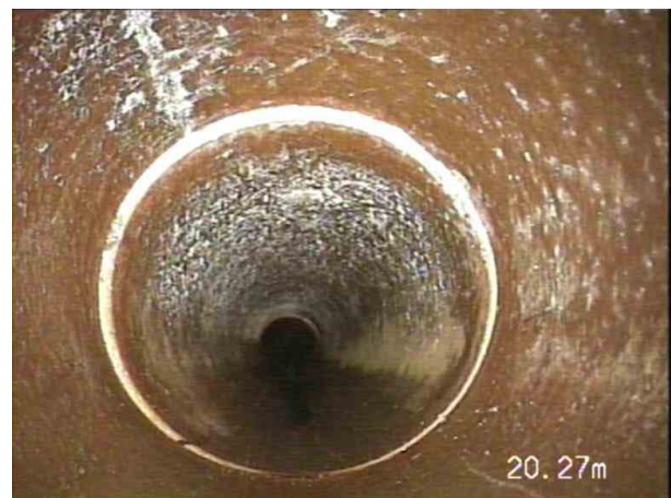
10, 00:03:46, 20.27 m Crack, longitudinal at joint at 5 o'clock
