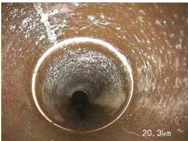
11, 00:03:39, 20.34 m Crack, longitudinal at joint at 11 o'clock
