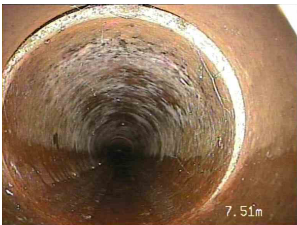
3, 00:01:15, 7.51 m Joint displaced, medium
