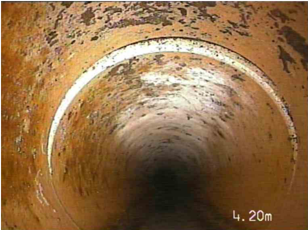
1, 00:00:52, 4.20 m Joint displaced, medium
