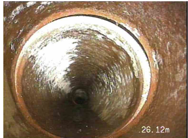
16, 00:04:52, 26.12 m Joint displaced, medium
