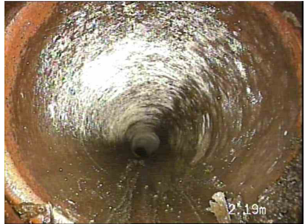
2, 00:00:44, 2.19 m Open joint, large
