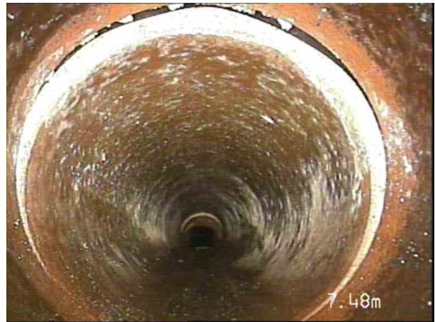
4, 00:01:33, 7.48 m Joint displaced, medium
