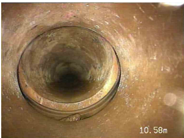
5, 00:01:55, 10.58 m Joint displaced, large
