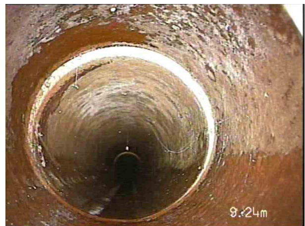
4, 00:01:31, 9.24 m Joint displaced, medium
