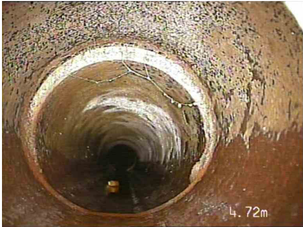
1, 00:00:41, 4.72 m Joint displaced, medium
