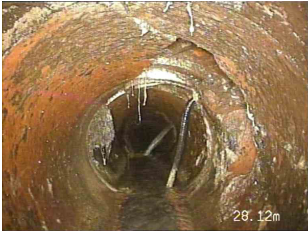
1, 00:03:28, 28.12 m Fracture, longitudinal at joint at 12 o'clock
