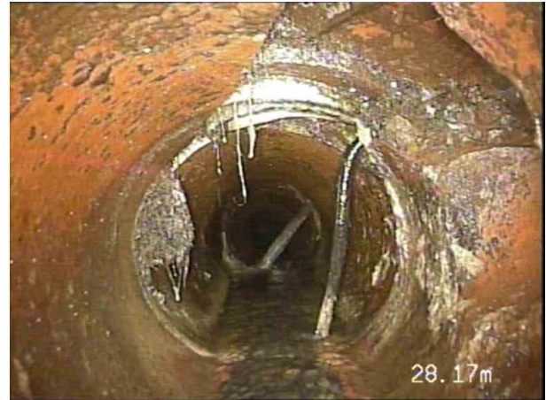
2, 00:03:41, 28.17 m Broken pipe from 11 o'clock to 1 o'clock
