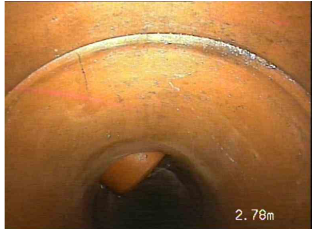
2, 00:00:38, 2.78 m Crack, longitudinal at joint at 11 o'clock
