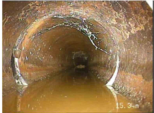
2, 00:02:01, 15.34 m Open joint, large
