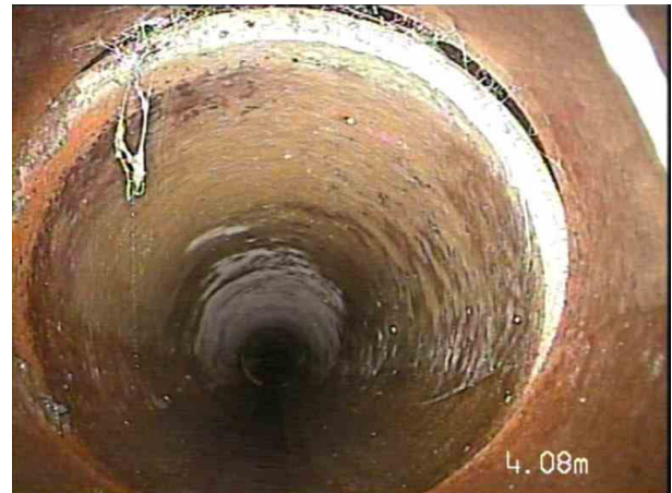
2, 00:00:50, 4.08 m Joint displaced, large
