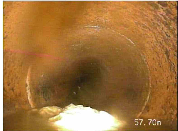
2, 00:11:01, 57.70 m Attached deposits, fouling from 5 o'clock to 7 o'clock, 25% cross-sectional area loss
