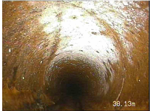
8, 00:04:48, 38.13 m Fracture, spiral from 11 o'clock to 5 o'clock
