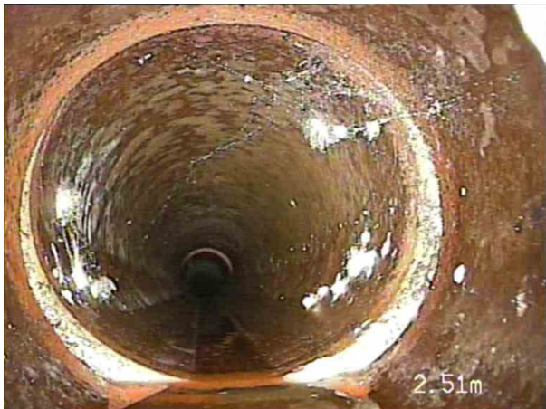
1, 00:00:33, 2.51 m Joint displaced, large
