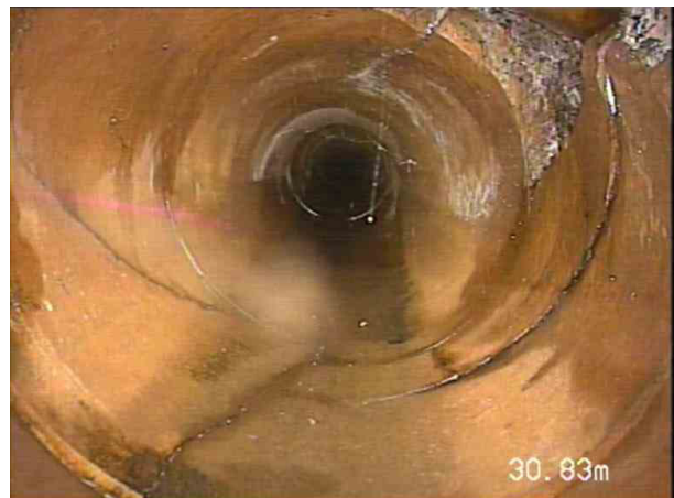
6, 00:04:46, 30.83 m Fractures, multiple from 2 o'clock to 12 o'clock
