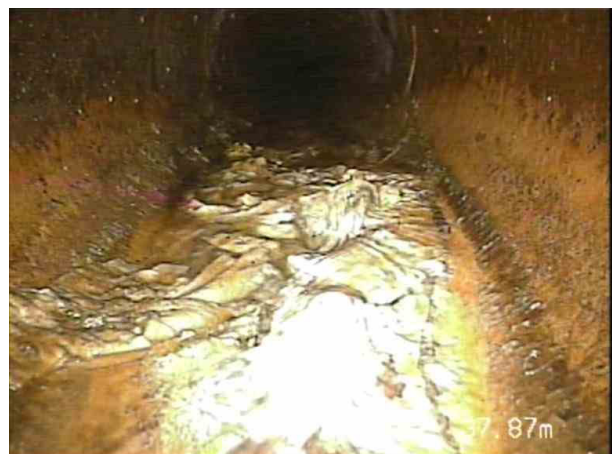
6, 00:04:31, 37.87 m Fracture, longitudinal at joint at 5 o'clock
