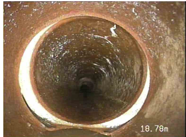
8, 00:03:23, 18.78 m Joint displaced, large
