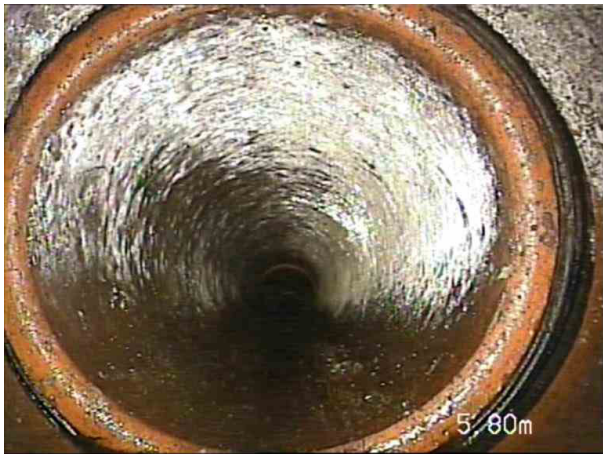
3, 00:01:18, 5.80 m Open joint, large
