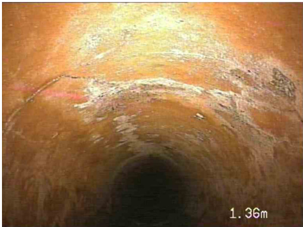
1, 00:00:42, 1.36 m Fracture, spiral at joint from 11 o'clock to 1 o'clock
