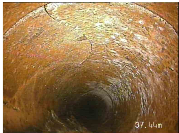
4, 00:04:04, 37.44 m Fracture, longitudinal at joint at 10 o'clock
