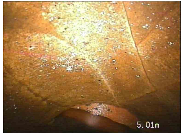
2, 00:01:04, 5.01 m Cracks, multiple from 1 o'clock to 4 o'clock
