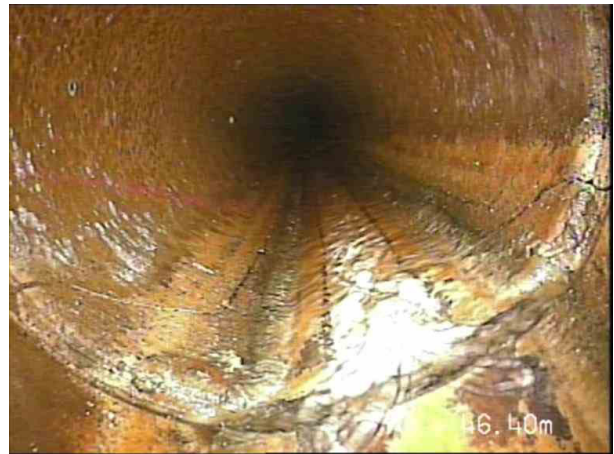
10, 00:05:47, 46.40 m Fracture, spiral at joint from 7 o'clock to 8 o'clock
