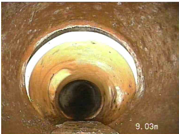
5, 00:01:47, 9.03 m Joint displaced, large
