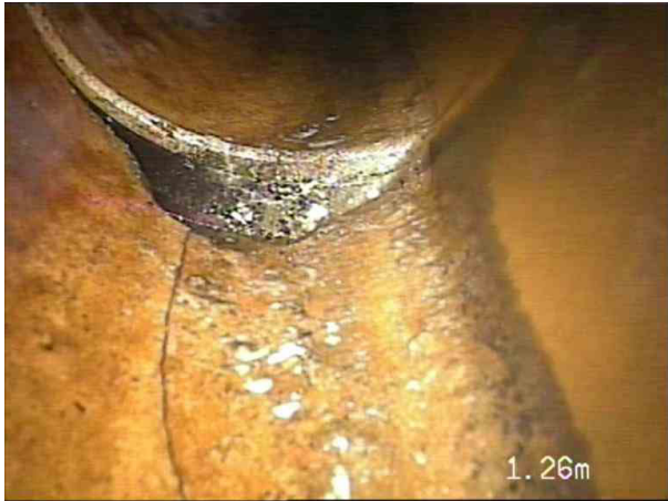
1, 00:00:28, 1.26 m Fracture, longitudinal at joint at 8 o'clock
