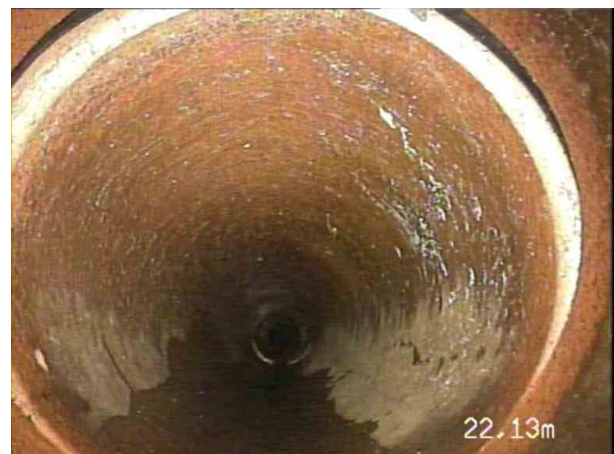
12, 00:04:06, 22.13 m Joint displaced, medium
