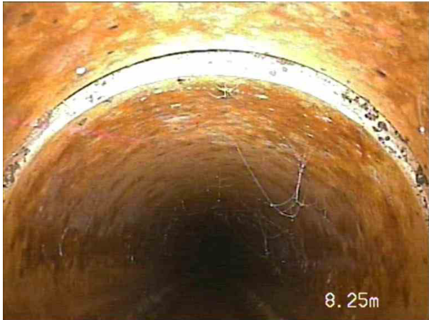
1, 00:01:12, 8.25 m Joint displaced, medium
