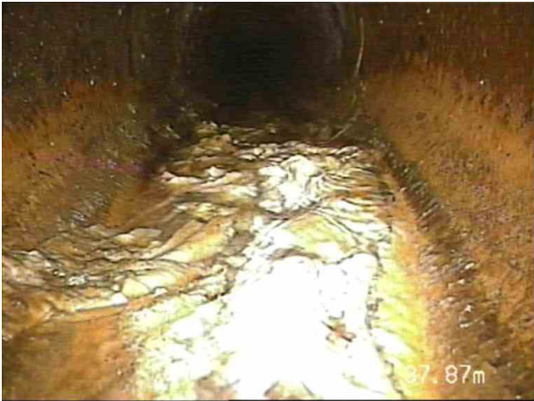
7, 00:04:33, 37.87 m Fracture, longitudinal at joint at 6 o'clock
