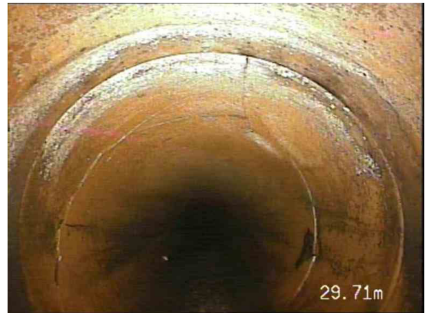
4, 00:04:41, 29.71 m Crack, longitudinal at joint at 12 o'clock
