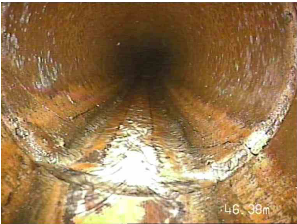
9, 00:05:40, 46.38 m Fracture, spiral at joint from 5 o'clock to 6 o'clock
