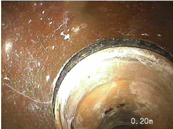
1, 00:00:13, 0.20 m Joint displaced, large
