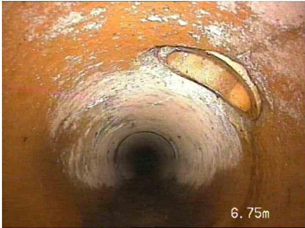
1, 00:01:11, 6.75 m Connection defective, connecting pipe is intruding at 1 o'clock, 100mm dia, intrusion: 5%
