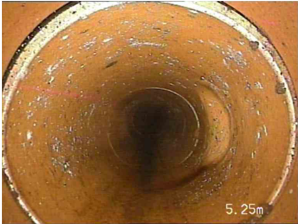
1, 00:00:47, 5.25 m Joint displaced, medium
