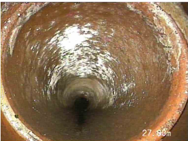
17, 00:05:05, 27.83 m Joint displaced, medium
