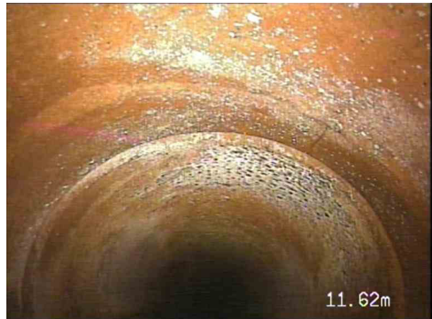
4, 00:01:52, 11.62 m Crack, longitudinal at joint at 1 o'clock
