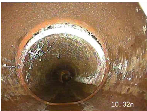
3, 00:01:52, 10.32 m Joint displaced, large
