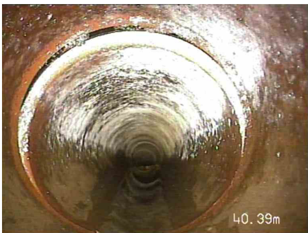
21, 00:06:50, 40.39 m Joint displaced, large
