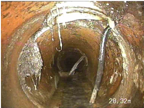
3, 00:03:51, 28.32 m Sealing ring intruding from 1 o'clock to 5 o'clock
