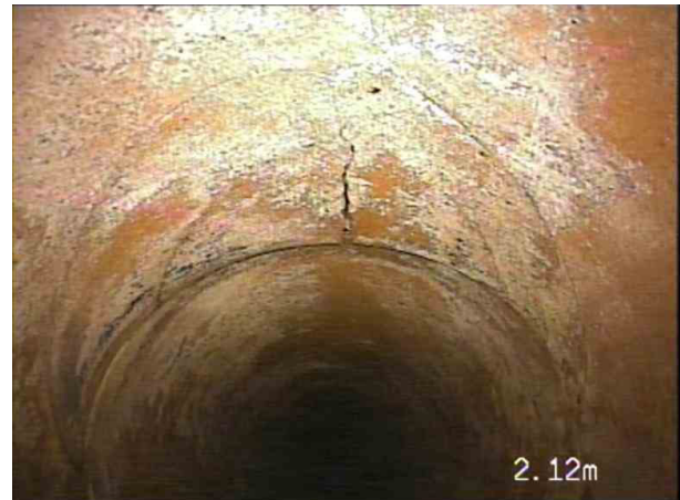
2, 00:00:55, 2.12 m Fracture, spiral at joint from 8 o'clock to 3 o'clock
