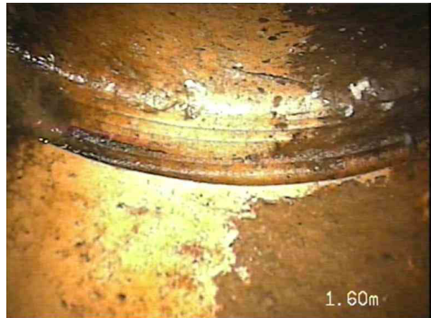
2, 00:00:35, 1.60 m Open joint, large
