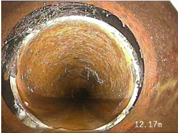
1, 00:01:39, 12.17 m Open joint, large
