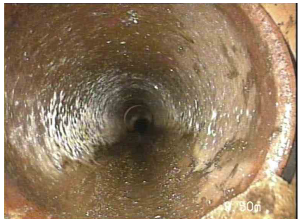
6, 00:02:03, 9.50 m Open joint, large
