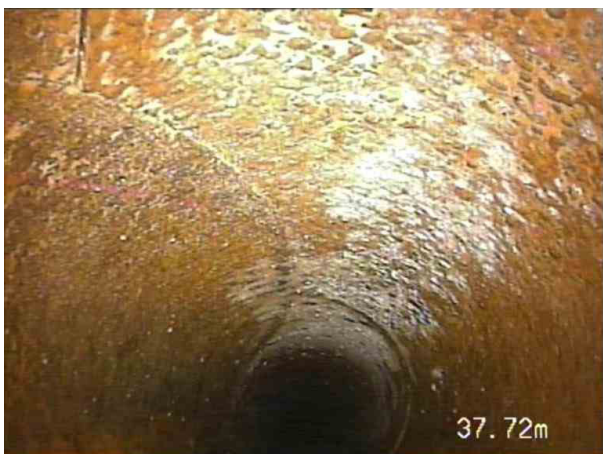
5, 00:04:18, 37.72 m Crack, longitudinal at joint at 11 o'clock
