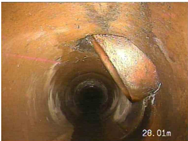
5, 00:03:54, 28.01 m Connection defective, connecting pipe is intruding at 2 o'clock, 150mm dia, intrusion: 20%
