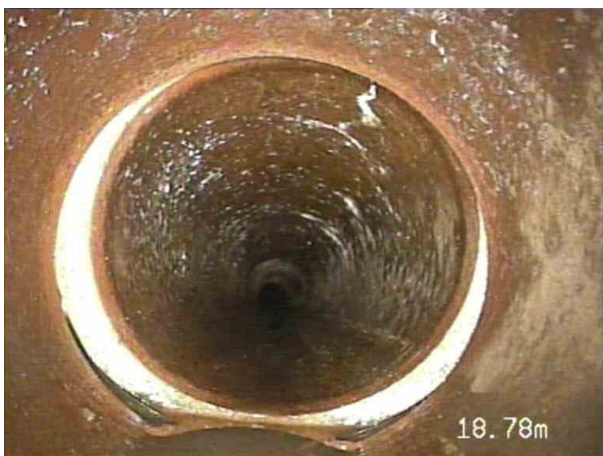
9, 00:03:26, 18.78 m Crack, longitudinal at joint at 1 o'clock
