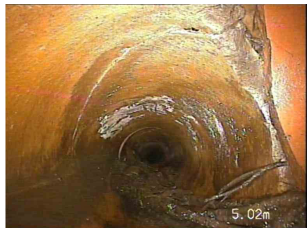
4, 00:01:18, 5.02 m Fracture, spiral from 8 o'clock to 1 o'clock
