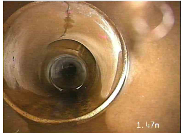
2, 00:00:27, 1.47 m Crack, longitudinal at joint at 12 o'clock
