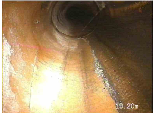
2, 00:02:46, 19.20 m Fracture, longitudinal at 9 o'clock
