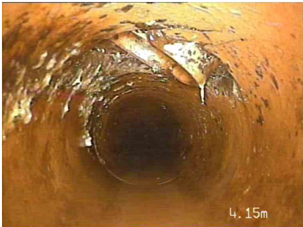
1, 00:01:09, 4.15 m Connection defective, connecting pipe is intruding at 12 o'clock, 100mm dia, intrusion: 5%
