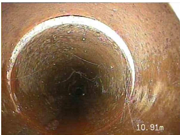
5, 00:01:44, 10.91 m Joint displaced, medium
