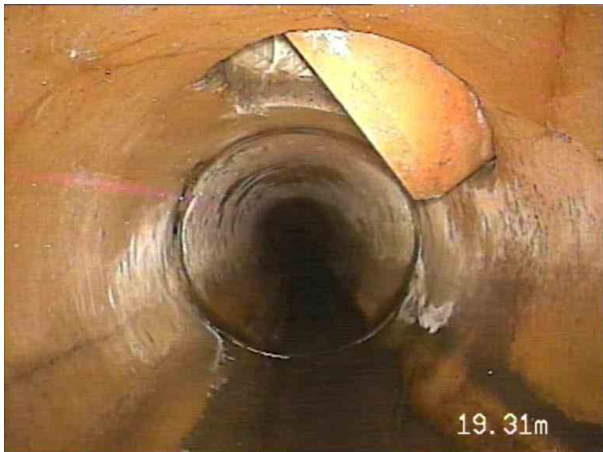
3, 00:02:53, 19.31 m Connection defective, connecting pipe is intruding at 1 o'clock, 150mm dia, intrusion: 15%
