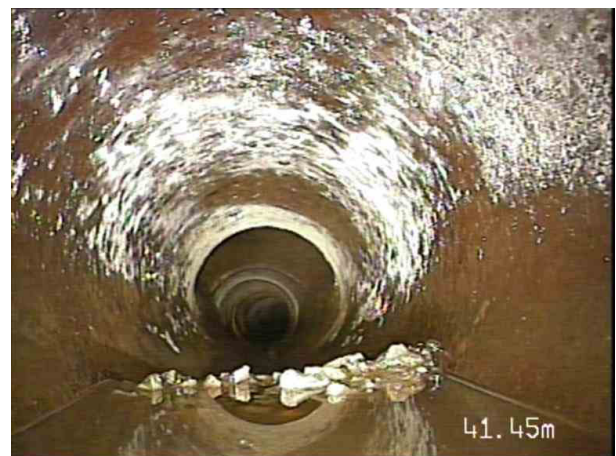
22, 00:07:04, 41.45 m Settled deposits, hard or compacted, 10% cross-sectional area loss, CONCRETE
