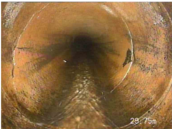
5, 00:04:48, 29.75 m Fracture, spiral at joint from 7 o'clock to 6 o'clock
