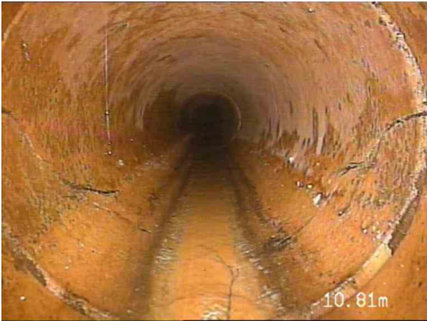
1, 00:01:17, 10.81 m Fracture, spiral at joint from 3 o'clock to 9 o'clock
