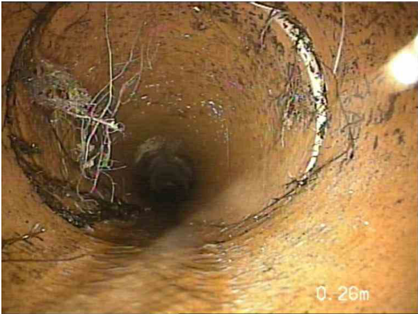
1, 00:00:18, 0.26 m Roots, tap at joint
