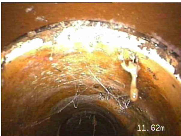
3, 00:02:57, 11.62 m Joint displaced, medium
