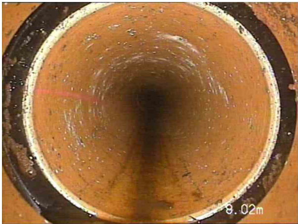
3, 00:01:22, 8.02 m Open joint, large
