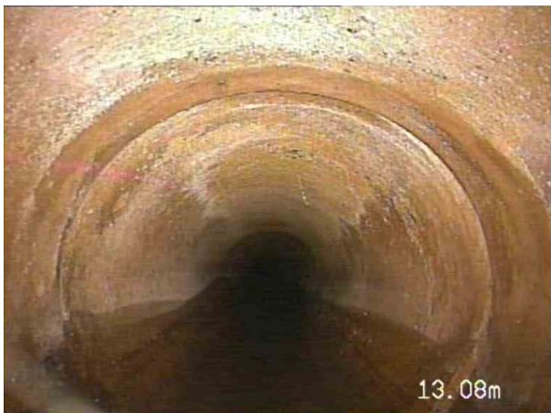
5, 00:02:07, 13.08 m Crack, circumferential at joint from 9 o'clock to 3 o'clock
