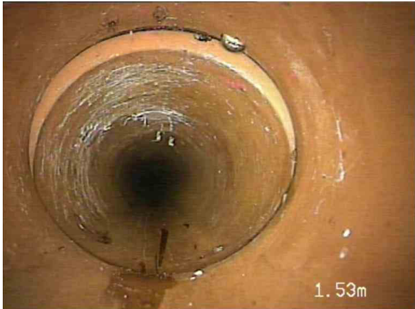
1, 00:00:26, 1.53 m Joint displaced, medium
