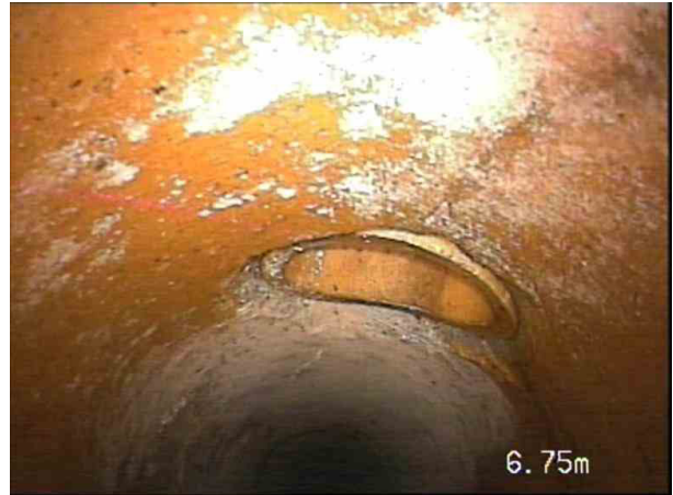
2, 00:01:16, 6.75 m Crack, longitudinal at 1 o'clock
