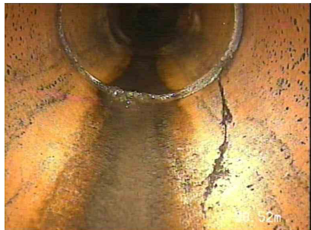
6, 00:05:03, 38.52 m Fracture, spiral at joint from 5 o'clock to 6 o'clock
