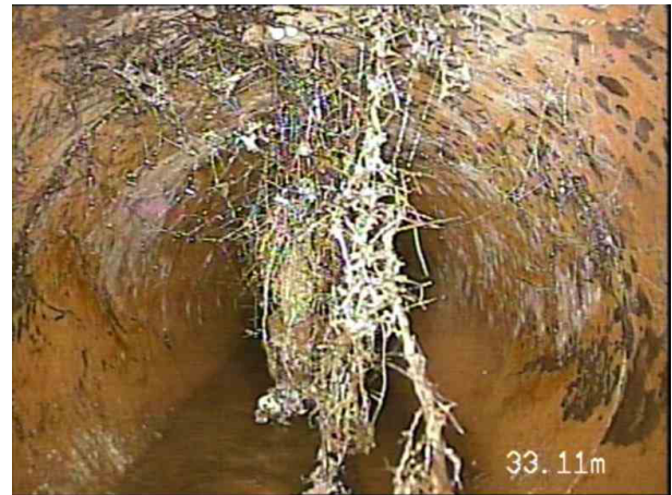
4, 00:04:58, 33.11 m Roots, mass at joint, 10% cross-sectional area loss
