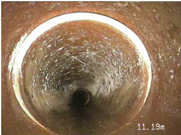
7, 00:02:22, 11.19 m Joint displaced, medium
