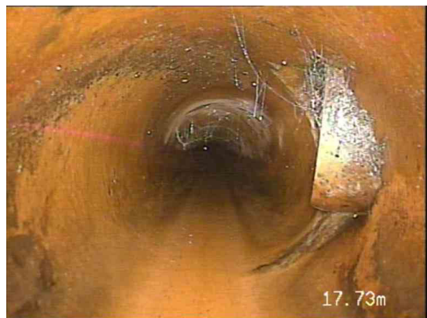
4, 00:04:06, 17.73 m Connection defective, connecting pipe is intruding at 3 o'clock, 100mm dia, intrusion: 10%
