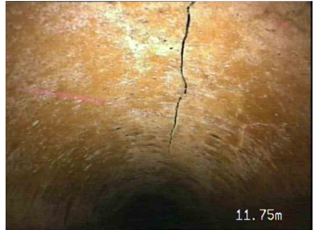
2, 00:02:19, 11.75 m Fracture, longitudinal at 1 o'clock
