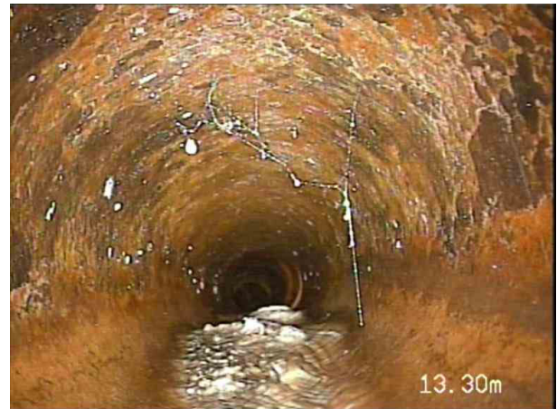
2, 00:02:00, 13.30 m Attached deposits, fouling from 5 o'clock to 7 o'clock, 10% cross-sectional area loss, LIVE LINE
