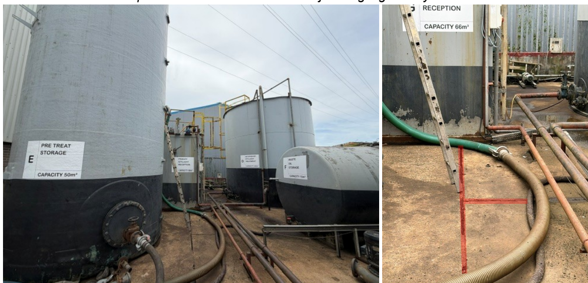
Figure 2 – LHS: Unsealed and open construction joints between concrete floor slabs adjacent to tanks D, E, F and G. RHS: A close up of the unsealed construction joint highlighted by the red line.
