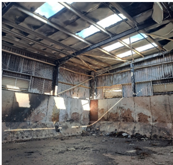
Image 1 shows the upper right hand corner of Building 1 which was the fire's origin point.
