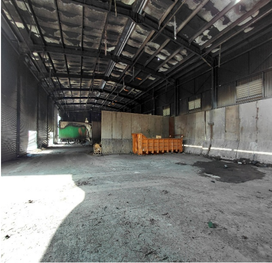
Image 3 shows wider view of Building 1, scorching along the roof is visible.
