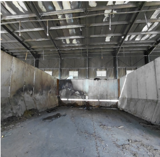
Image 4 shows the bay in Building 1 that has been used for green waste. Since the fire, green waste is now managed in Building 2 until permanent arrangements can be finalised.
