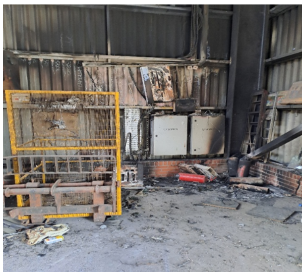
Image 2 shows the electrical power boxes for Building 1 which were damaged during the fire, resulting in a loss of power to Building 1.
