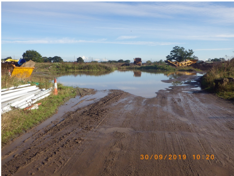
Standing water on site
