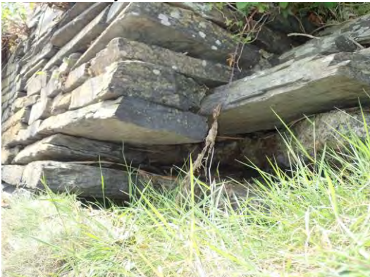
Plate a Cavity at base of wall
