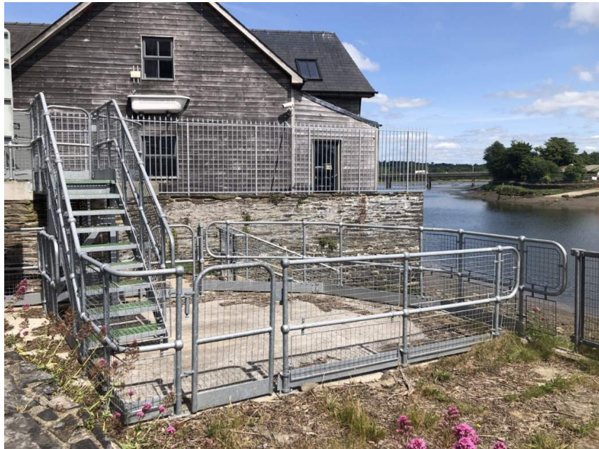
Figure e-3 – Dŵr Cymru Welsh Water discharge chamber (ID: 146).
