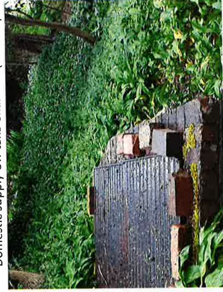
Domestic supply Off-take Chamber (Photo 5)
