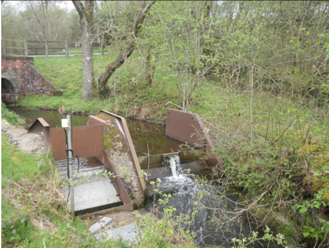
Blockage in hands off flow and residual flow notch whilst abstraction taking place.
