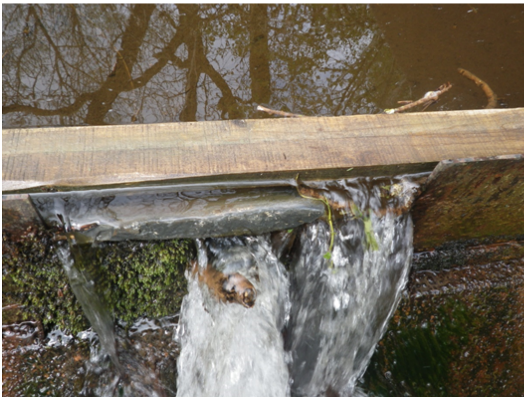
Blockage in residual flow and hands of flow notch.
