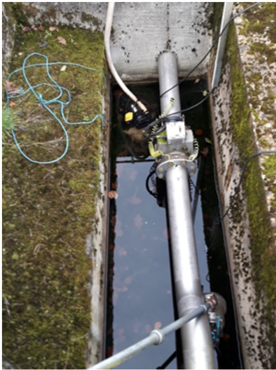
Photo 2: In pipe Magflow meter.
