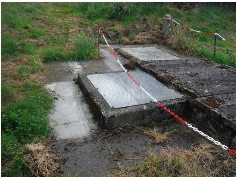
Photo 1: Evidence of a leak from the reed bed or the septic tank structure.
