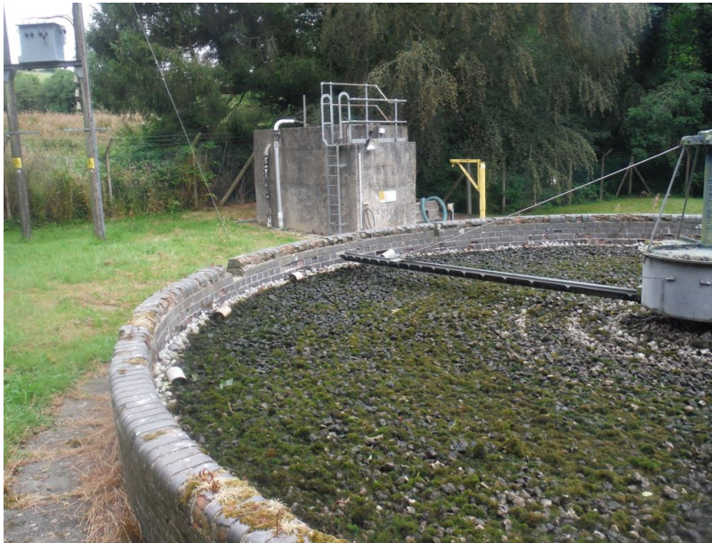
Photo 1: Missing and crumbling brick work on filter bed wall.
