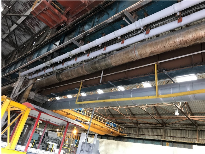
Overhead guttering collecting hydraulic oil from parked overhead crane.
