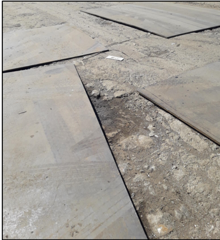
Image 1 – showing weakened infrastructure in need of repair, covered with metal sheets for plant on site – taken on 13/08/19
