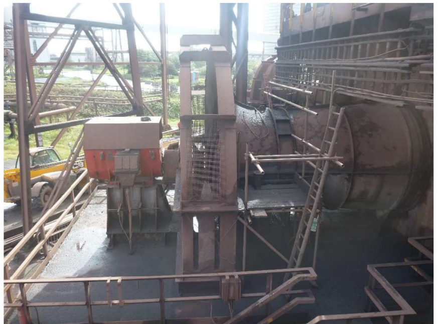
Photograph showing number 2 cooler fan. Sound abatement scheduled for installation w/c 19 th September.
