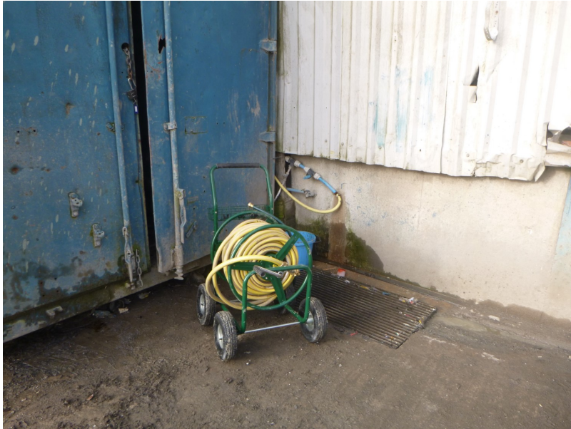
Photo of the fire hose provided by the site
