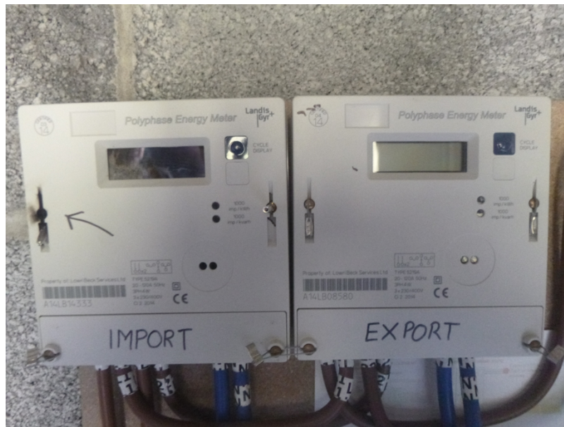
Figure 2: The meters in the Turbine House.
