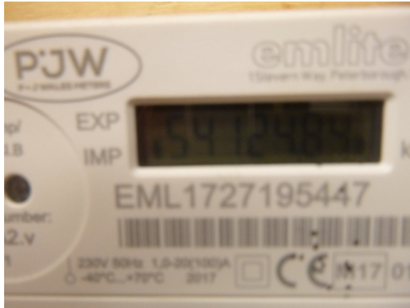
Figure 2: The meter in the Turbine House
