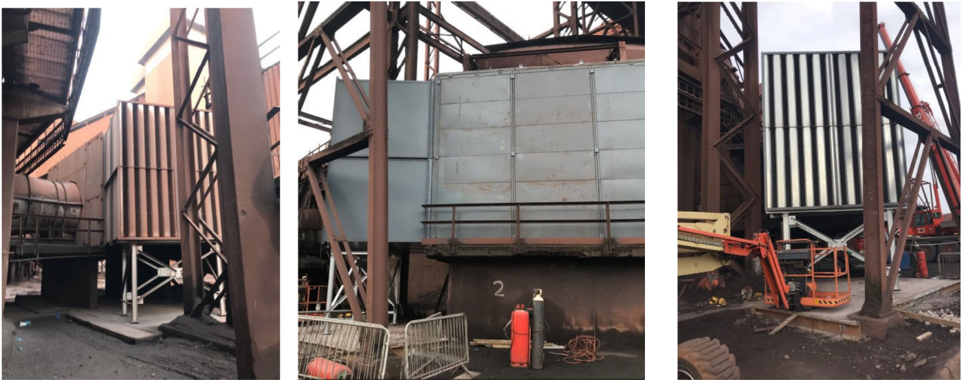
Photographs showing new noise abatement enclosures in place on some of the Sinter Plant Cooler Fans
