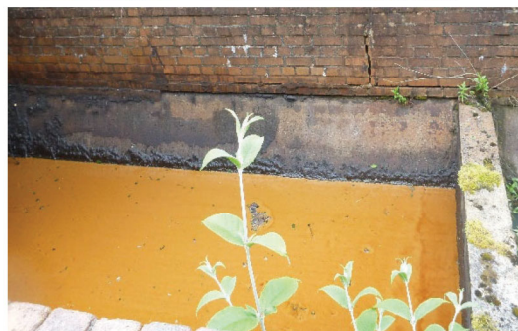
SW Interceptor June 2017 – significant contamination in surface water interceptor.
