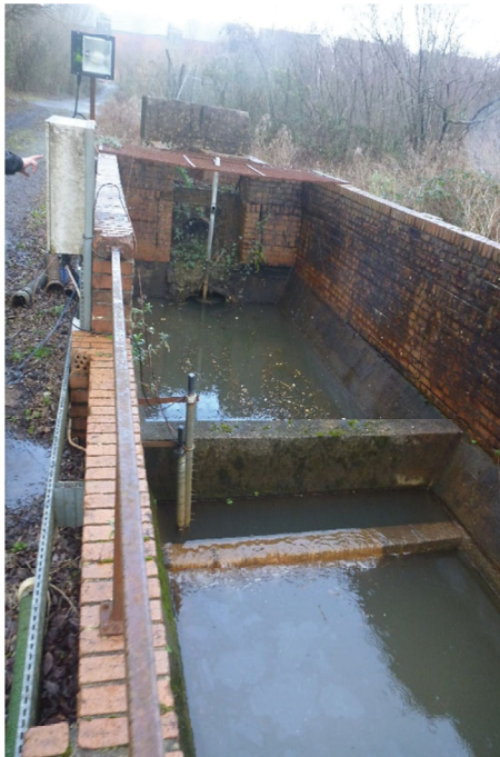
SW Interceptor February 2020 – no evidence of major contamination. Vegetation cleared
