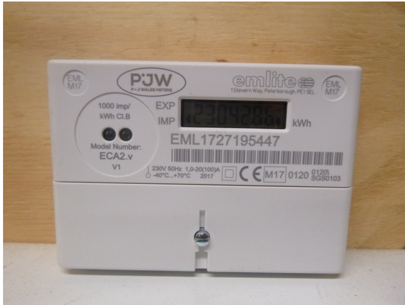
Figure 2. The meter in the Turbine House.
