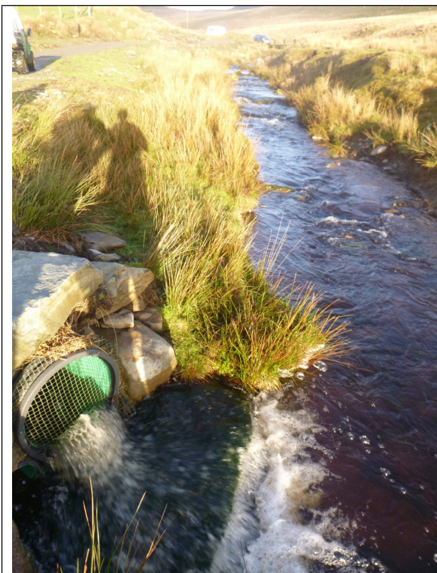
Figure 3. The outlet pipe into the Nant y Mean.
