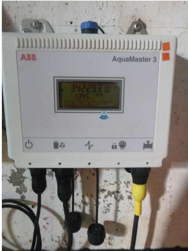
Figure 2. Water meter at Llyn Egnant.
