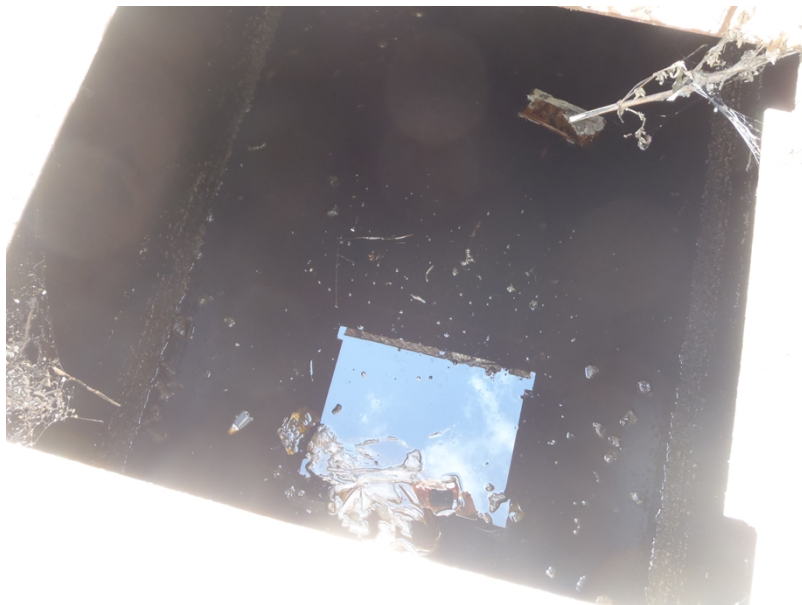
Inside the metal oil interceptor
