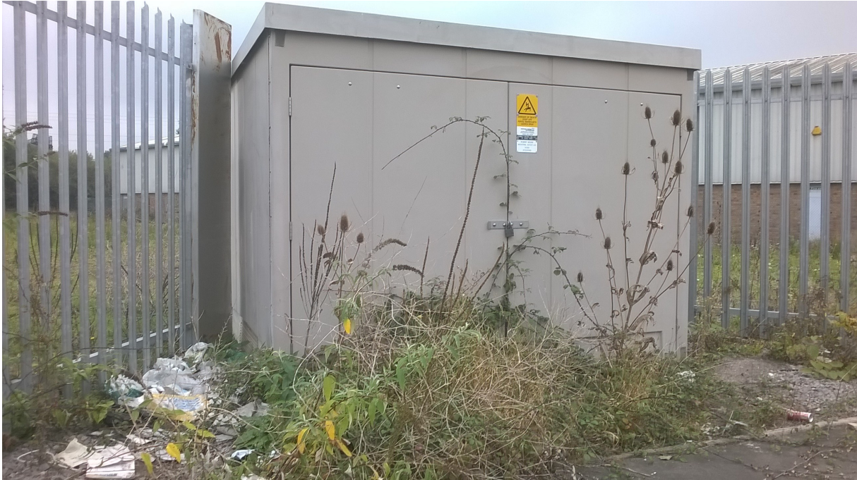
Photo 5— Electricity substation along southern boundary.
