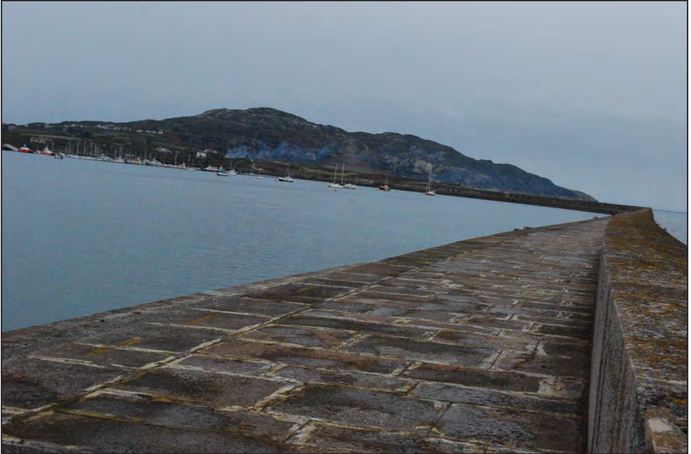
Plate 15: Holyhead Breakwater - view from east looking towards Holyhead mountains from upper parapet (archive image: G2498_042).
