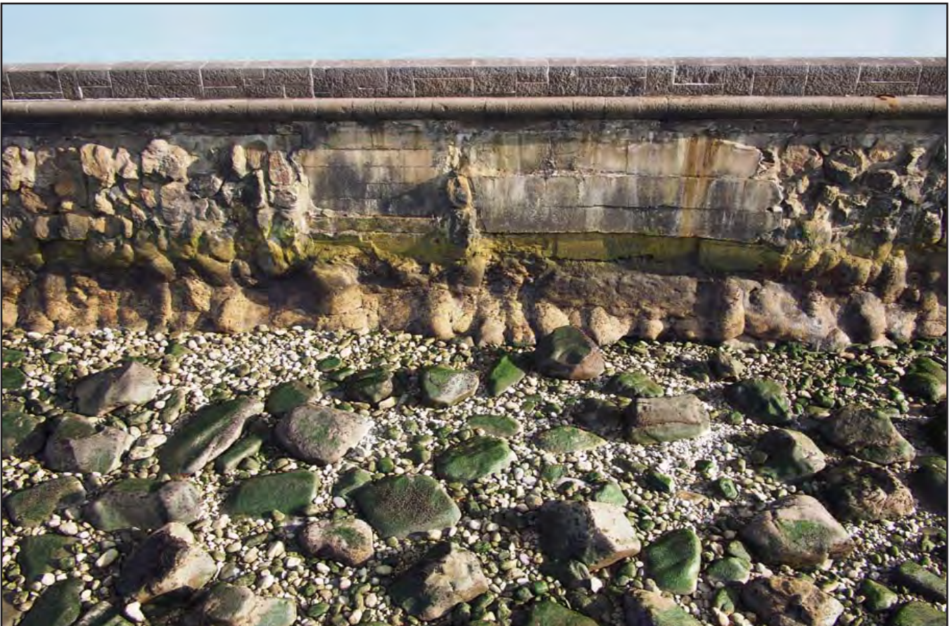
Plate 08: View of further concrete repair work along seawards side of the breakwater (sourced from Civil Engineering Solutions: 20150928 Holyhead Breakwater 203.jpg).
