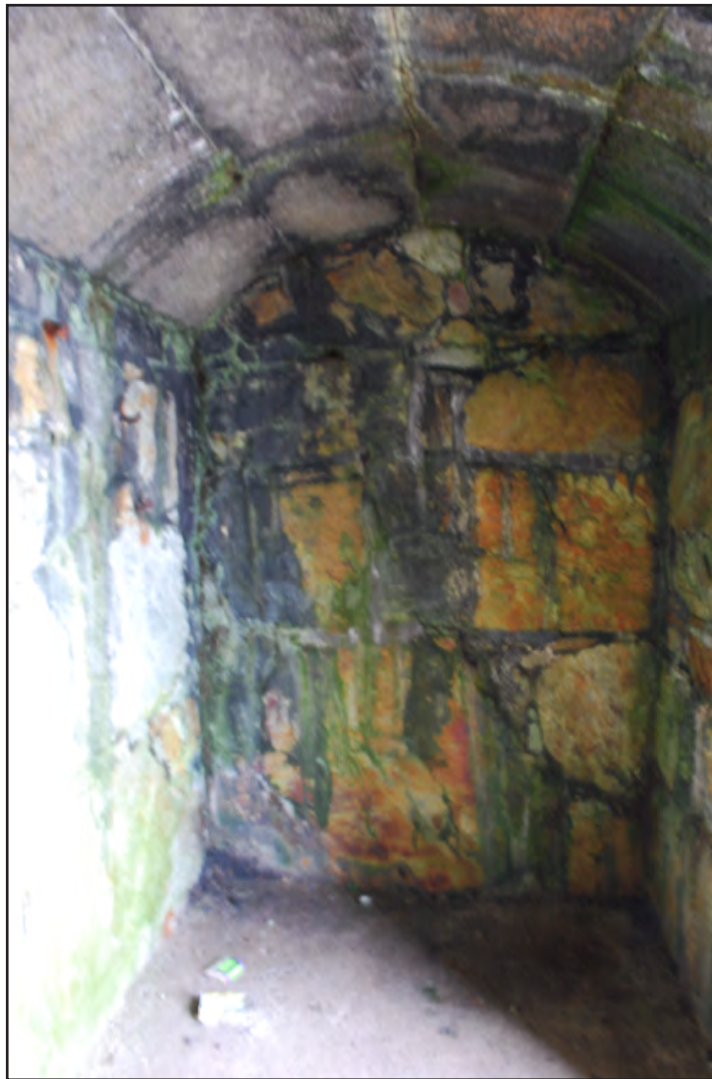
Plate 19: Holyhead Breakwater - interior view of barrel vaulted refuge chamber (archive image: G2498_009).
