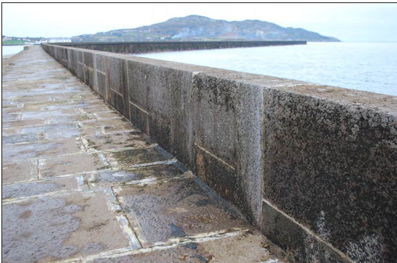
Plate 26: Holyhead Breakwater - view from southeast of parapet ashlar showing cyclopean blocks (archive image: G2498_037)
