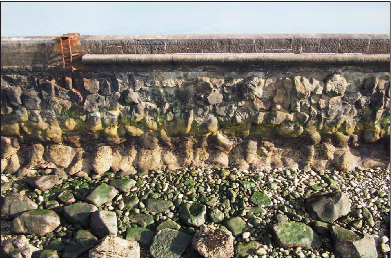
Plate 06: Seaward view of parapet with the remnants of a later addition of a ladder, possibly used in emergencies (sourced from Civil Engineering Solutions: 20150928 Holyhead Breakwater 206.jpg).
