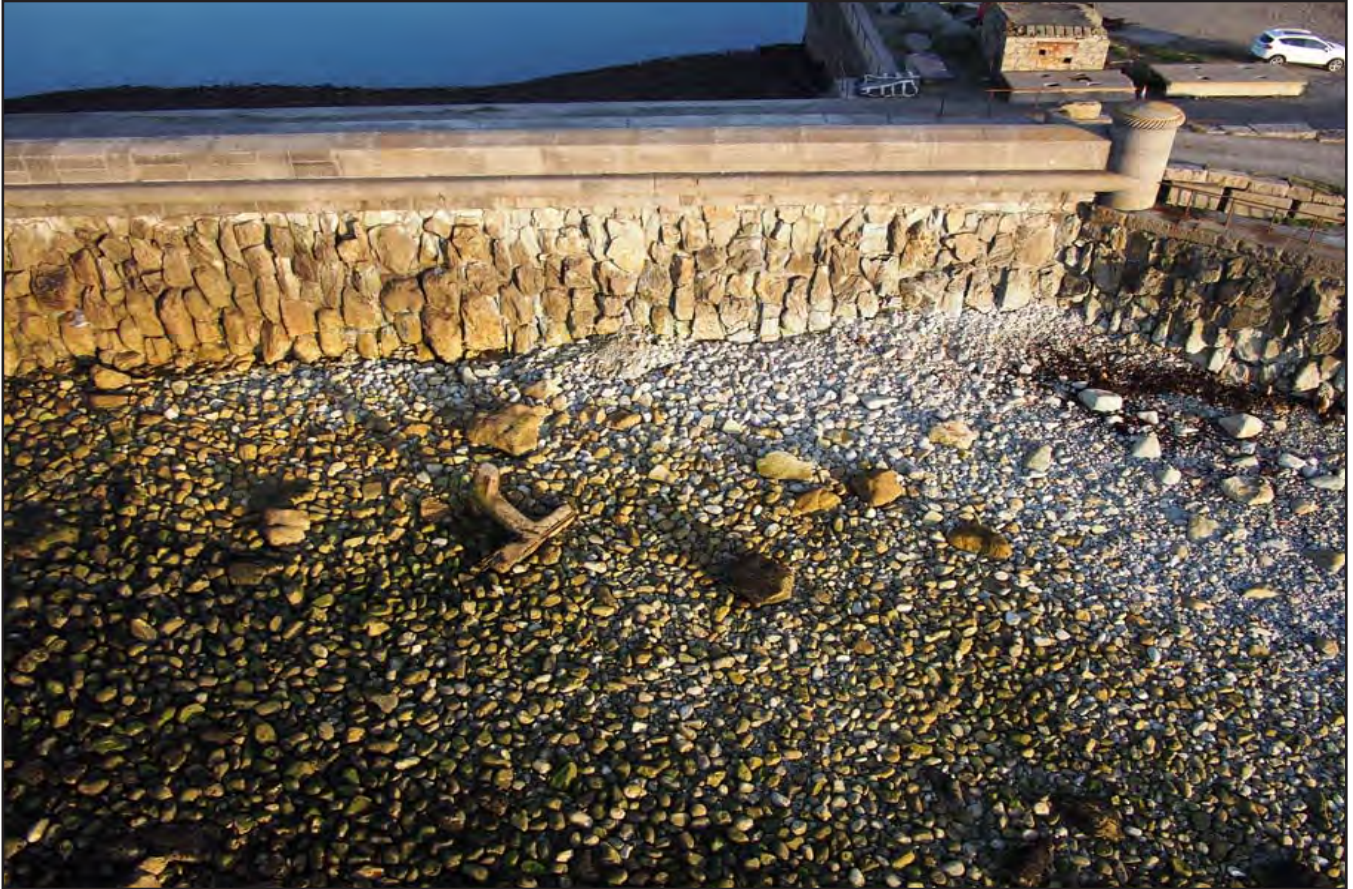
Plate 03: Seward view of the parapet at landsend, showing large rubble foundation blocks supporting the parapet (sourced from Civil Engineering Solutions: 20150928 Holyhead Breakwater 1086.jpg).
