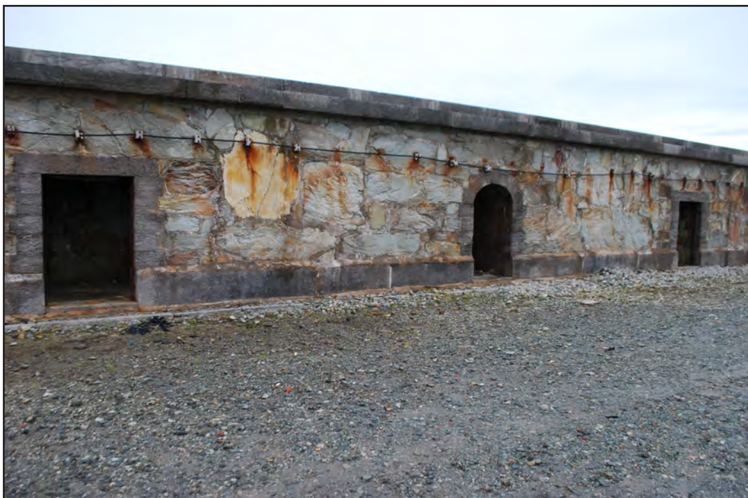
Plate 20: Holyhead Breakwater - view from southwest of three barrel vaulted refuge chambers (archive image: G2498_010).
