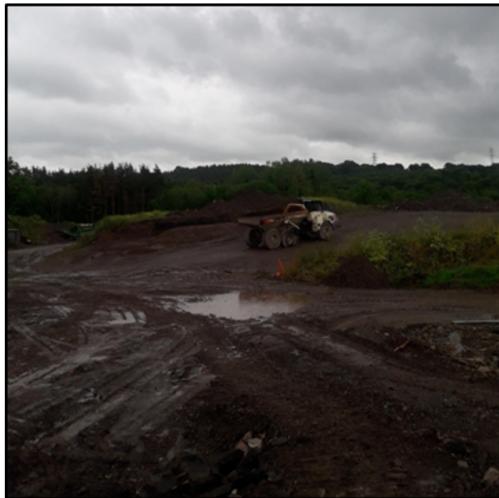
Image 2 – showing where the stockpiled had been levelled out.
