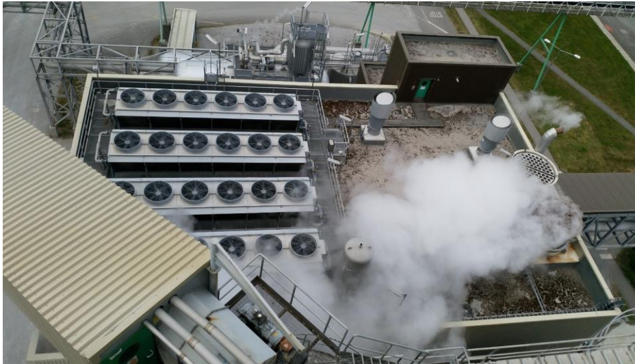
Figure 3-6 – Dry air coolers
