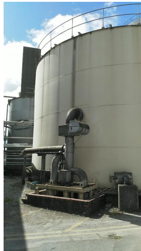
Fresh water pipe
