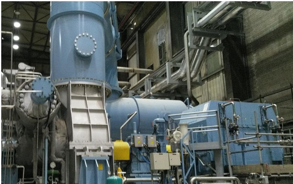
Figure 4-2 – Low pressure condensing turbine hall
