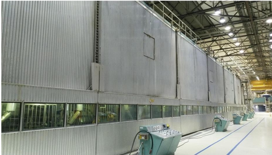
Figure 4-1 - Enclosure over dryer hood to reduce noise emissions (PM2)
